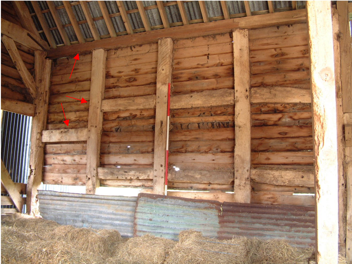
Plate 5: General pattern of framing as viewed in bay 1 northern side. Timbers arrowed are later insertions, see Plate 6 (scale 2-metres)
