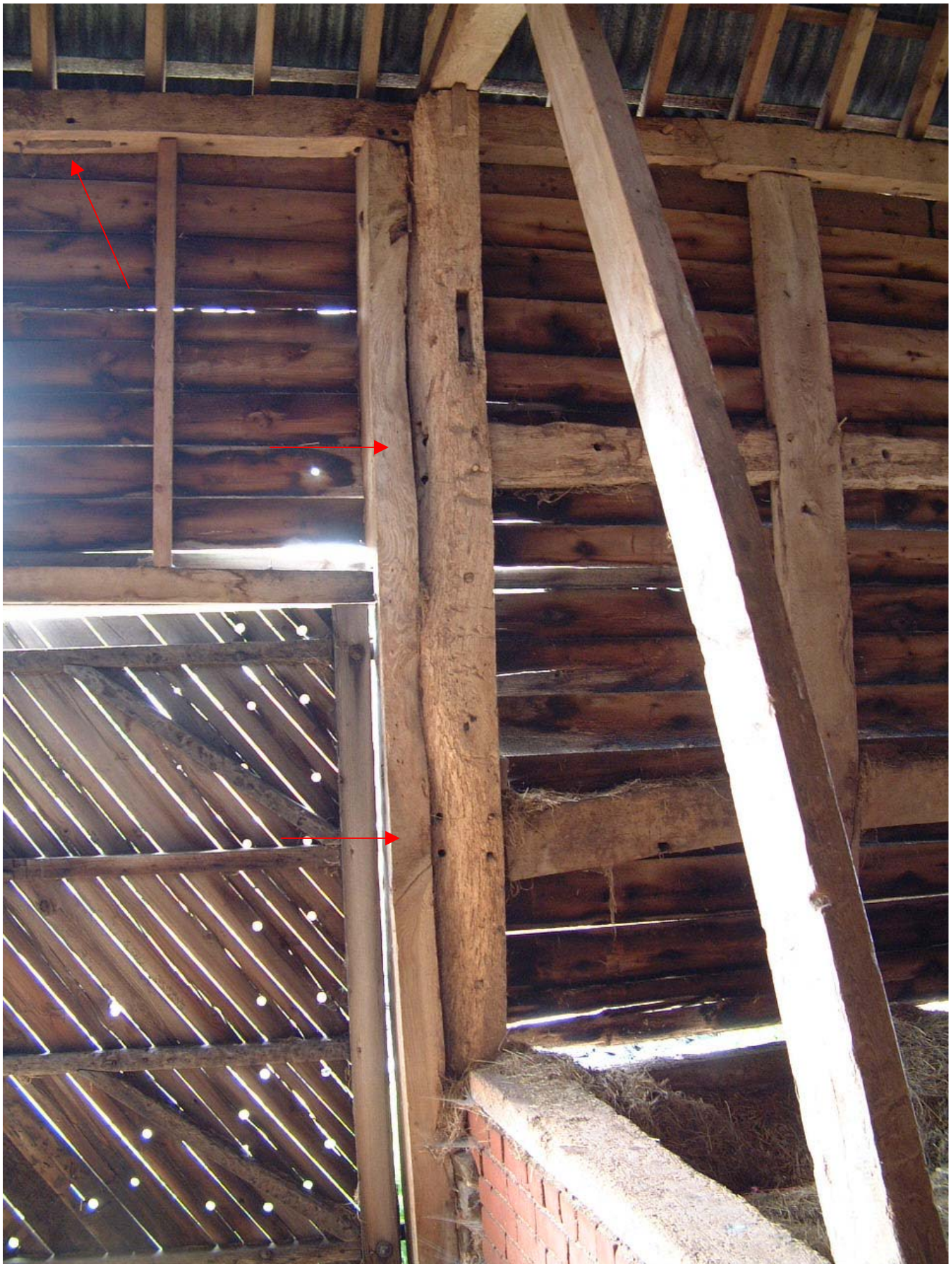
Plate 15: Empty mortises and peg holes in T2 south side and wall plate (arrowed) indicating framing extended across the present cart bay.
