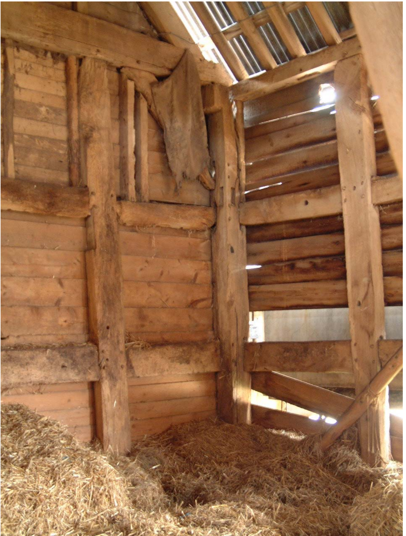
Plate 16: South-east corner post showing 'modified' head and empty mortises for bracing
