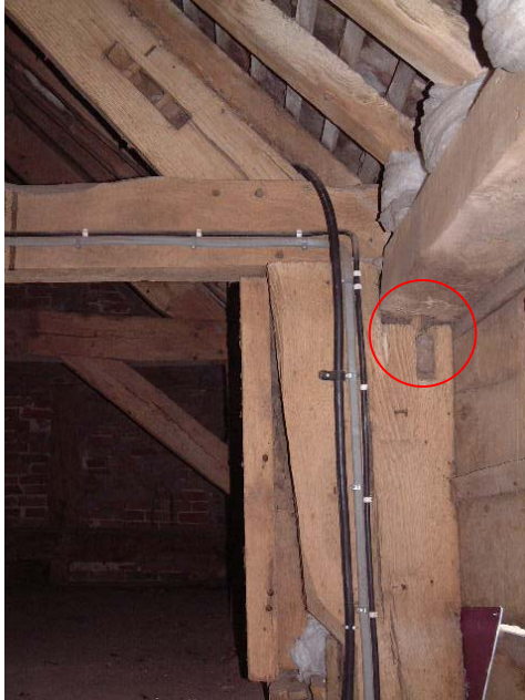
Unusual slip tenon at top of post indicating modification to the original
