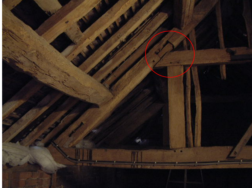
Original position of the clasped purlin at the collar, note the crack in the principal above
