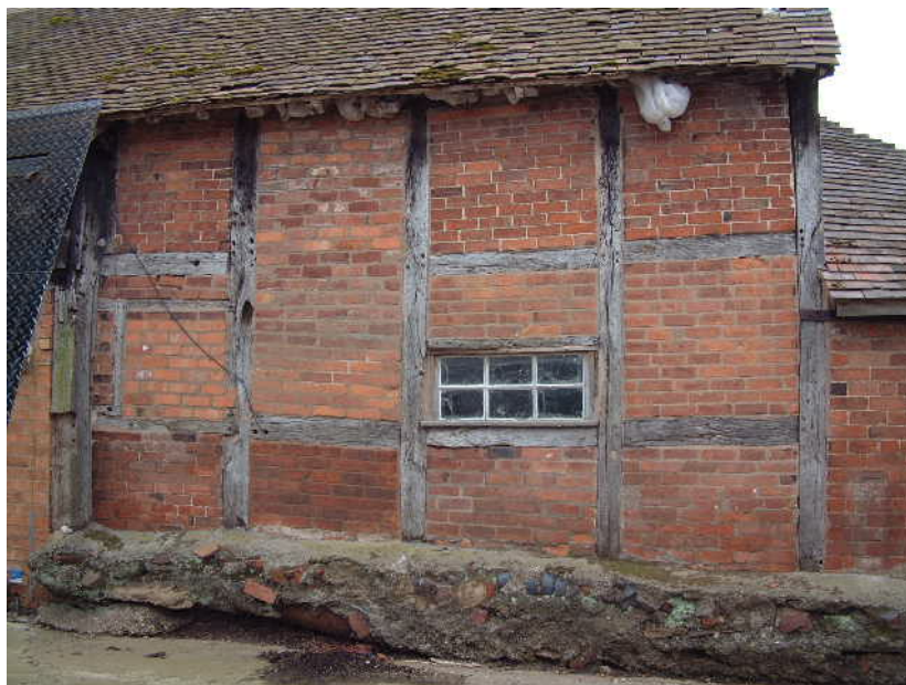
Northern elevation frame of the attached (chop house) building. The end post (right) has no visible carpenter's mark, but the next 3 (right to left) are marked I, II and III
