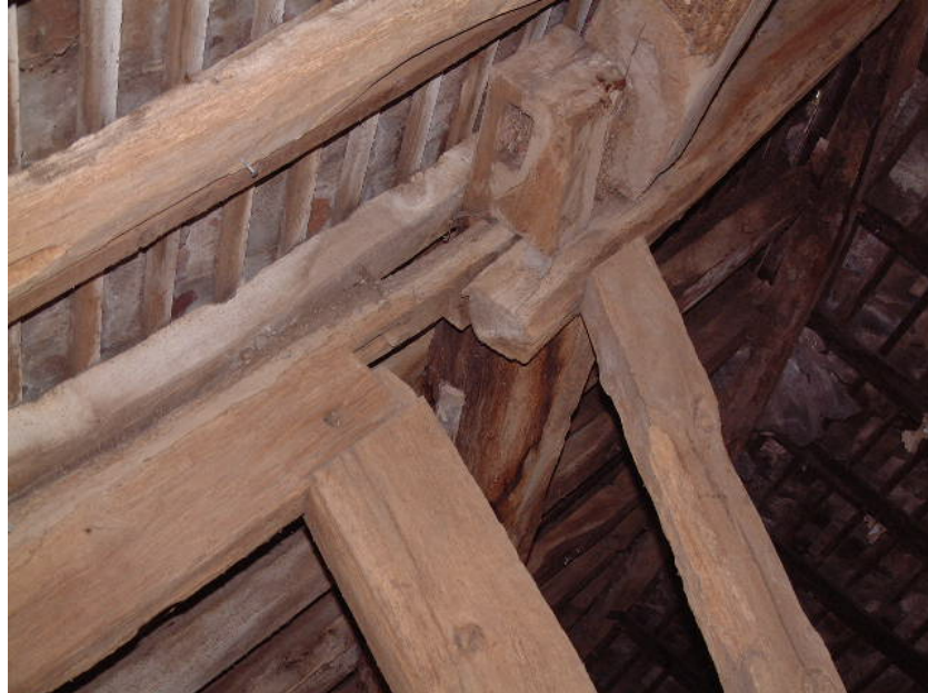
Top end of principal shown wedged up, as removal of the clasped purlin has caused it to crack
