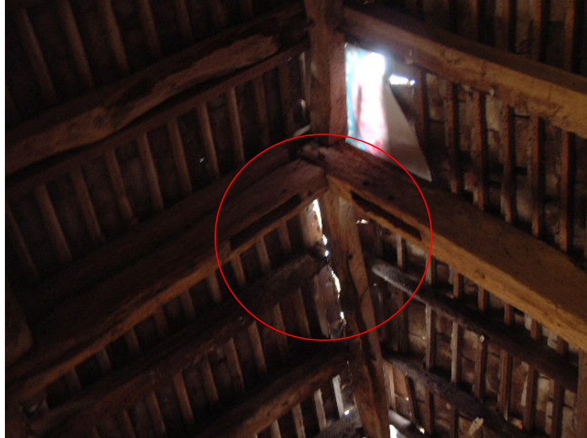
Empty mortises at top of truss showing position of a block, which was probably removed when the new trenched purlins were added
