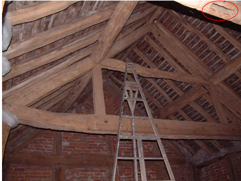
Central truss in chop house. Note the empty mortise on the base of T4 tie-beam, where the end frame has been removed (ringed).
