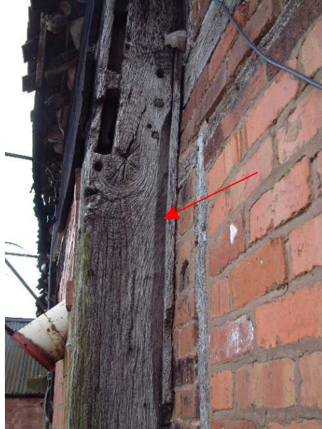
NW corner post of the barn (truss T4) showing the chamfer on the outside (arrowed)
