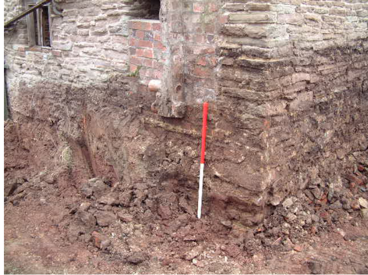
The level of build up against the building, note the bricked up window (scale 1 metre)
