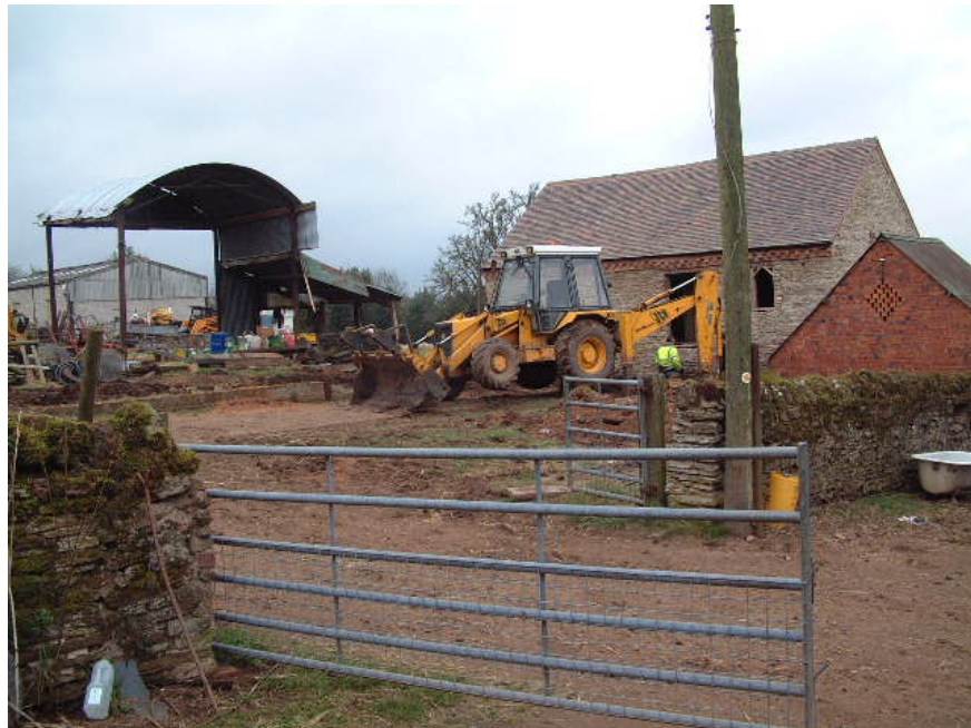
Work in progress. Note the Dutch barn (left). It is proposed that the dumped material was to facilitate a level platform for its construction
