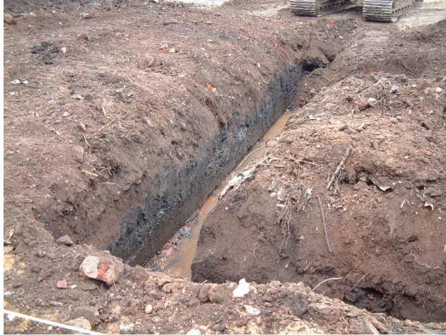
Waterlogging on the eastern side of the site
