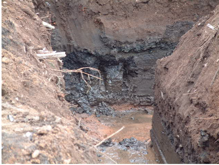
Waterlogging within the backfill of the pond at its eastern side
