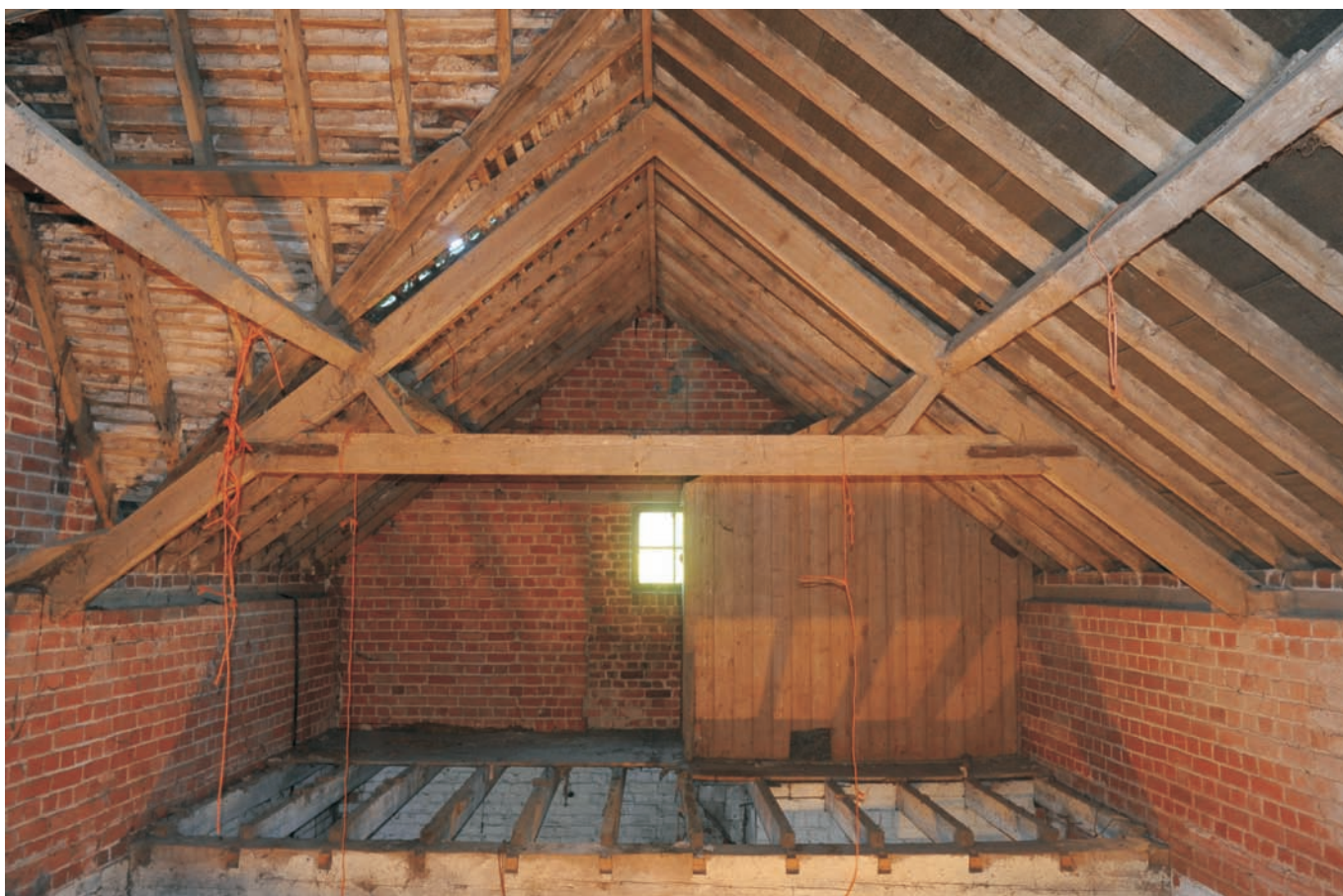
Northern end of upper floor of "Root House, showing matchboarded enclosure of inserted staircase"
