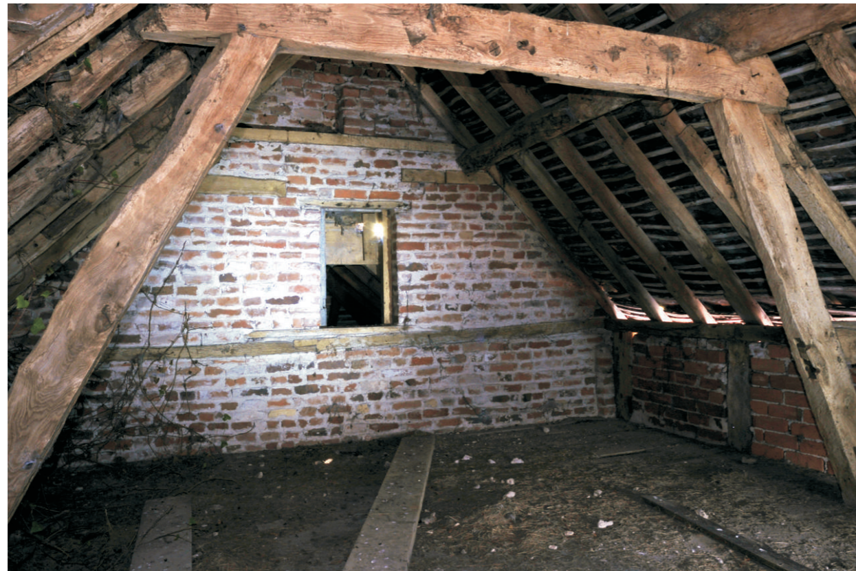
Western end of hayloft - note former opening blocked by construction of western stable roof
