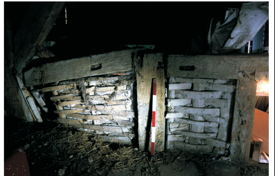
Detail of woven infill panels in internal partition wall at hayloft level
