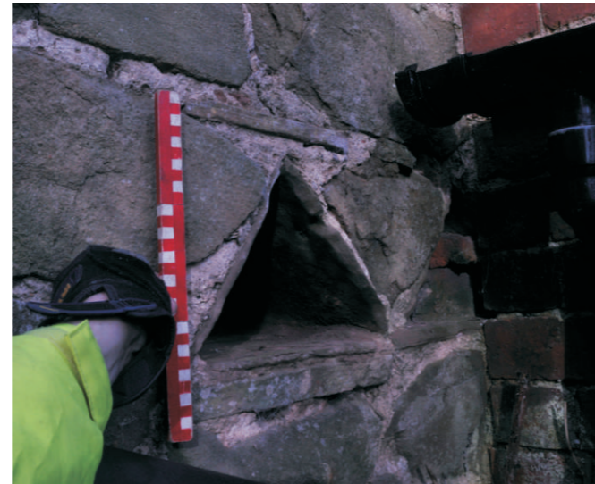
Detail of vents blocked by tack room extension
