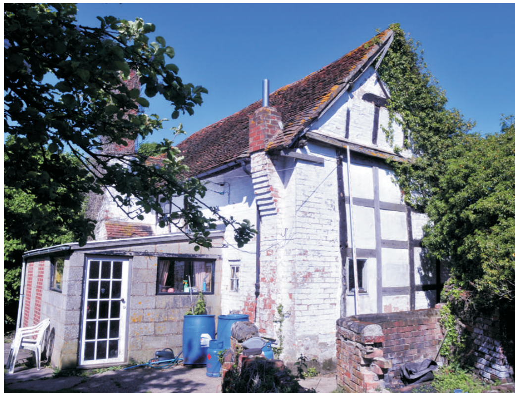
View from south east, note partially restored framing, and unsightly lean-to
