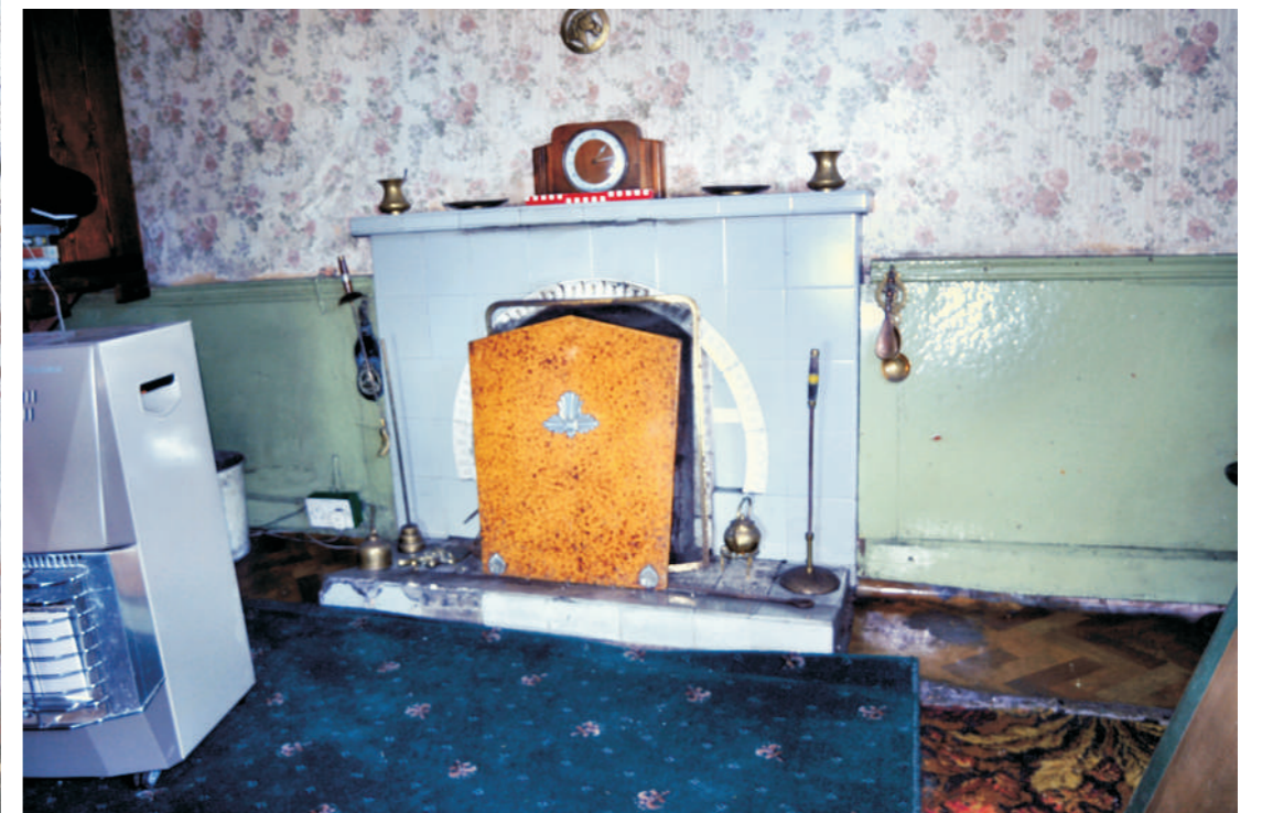
Inserted fireplace (1950s) on western gable end wall, note also modern ?fibreboard panelling to dado level
