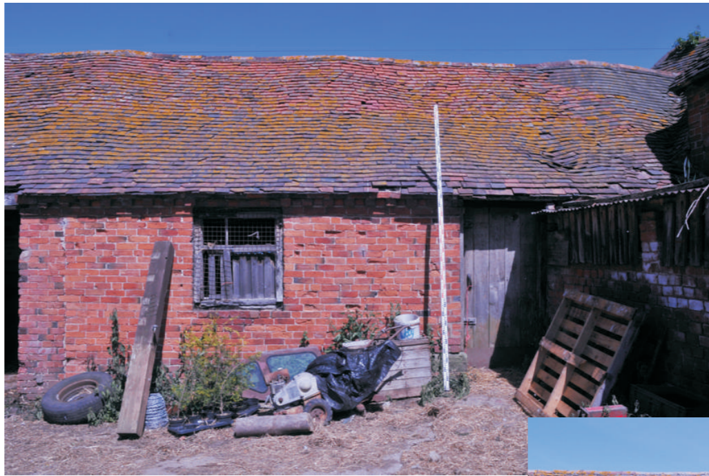
Shelter building northern side of foldyard, adjoining the barn - of 18th C origins with later modifications
