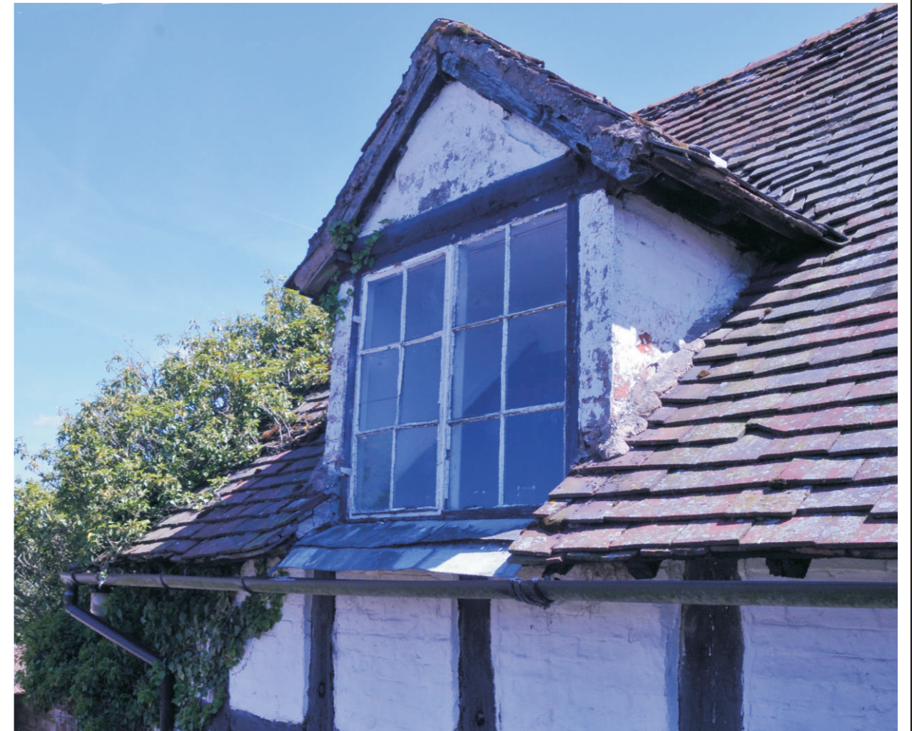
Detail of dormer, note fine early 19th C casement window, and brick construction of cheeks
