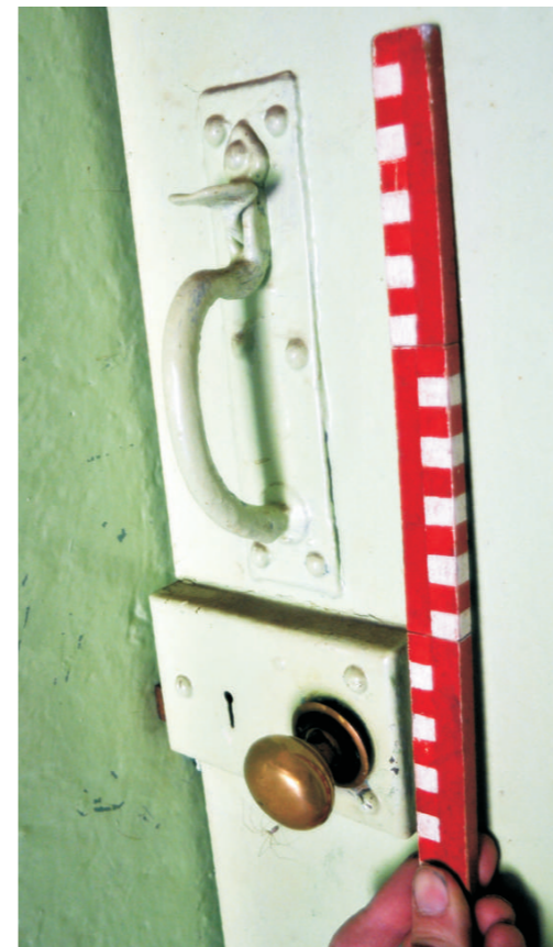
Detail of mid 19th C latch lifter and lock to stair door
