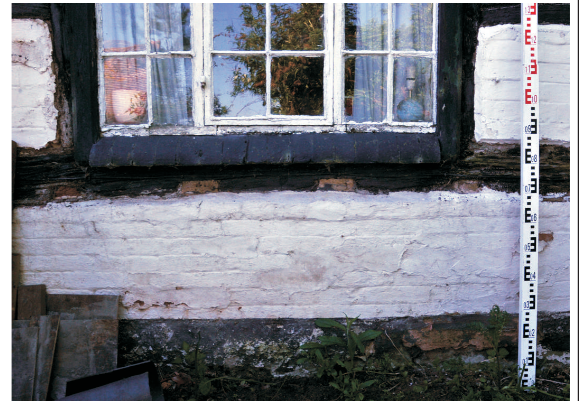
Detail of plinth wall - note that ground cill of framing is re-used timber
