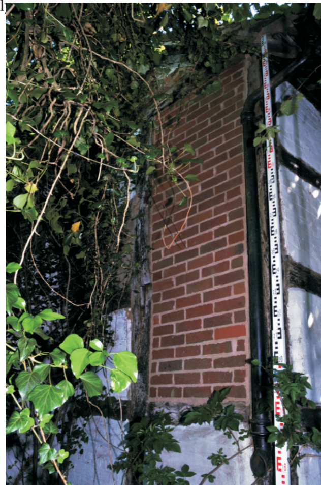
Detail of recent inappropriate repair to western gable
