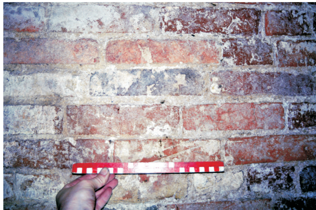
Detail of brickwork northern wall of cellar - brick is of late 17th-very early 18th C date. Brick size 220x53x105mm.
