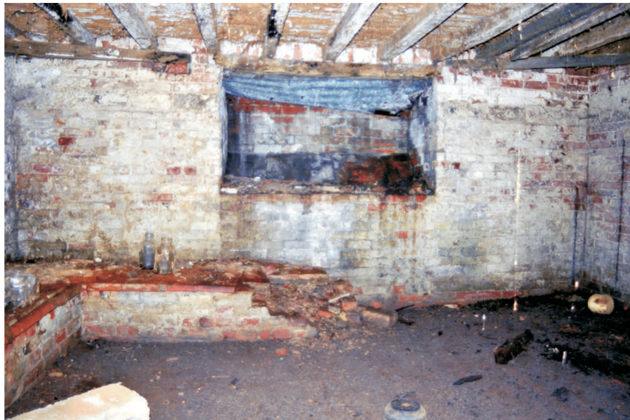
Southern wall of cellar, note brick built stillage and blocked access
