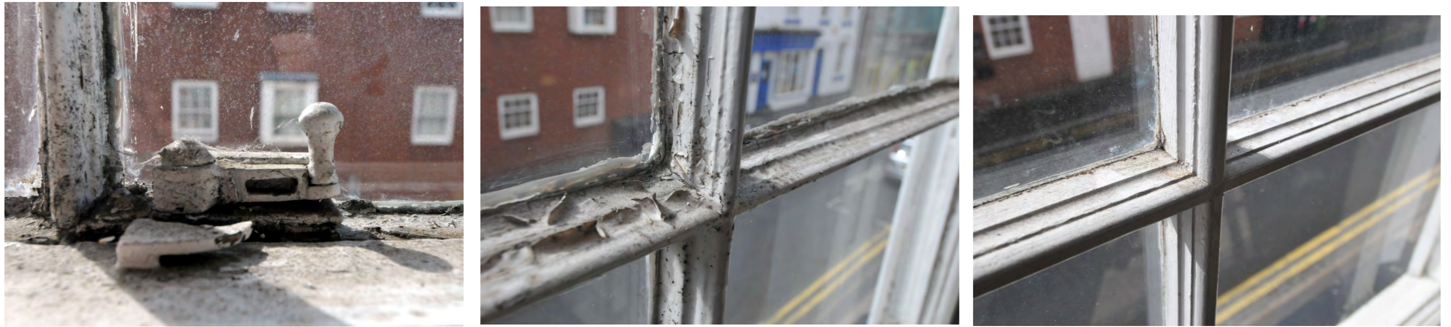
Window details front elevation 1st floor showing original glazing bar and replica profile ( above)
