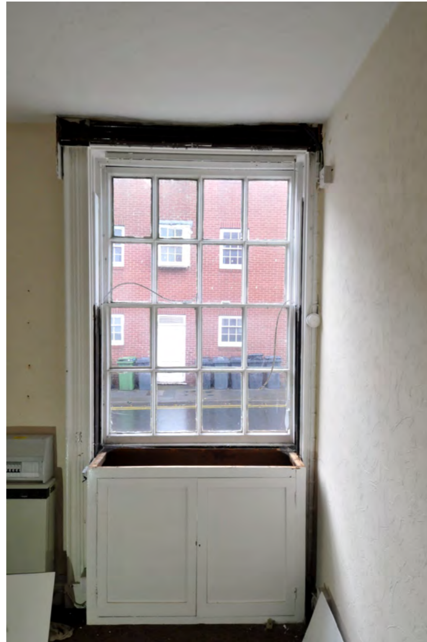
Window to front elevation - note that the window is both off-centre and partially obscured by partition wall. Cupboard is later addition replacing original vertical sliding shutter box
