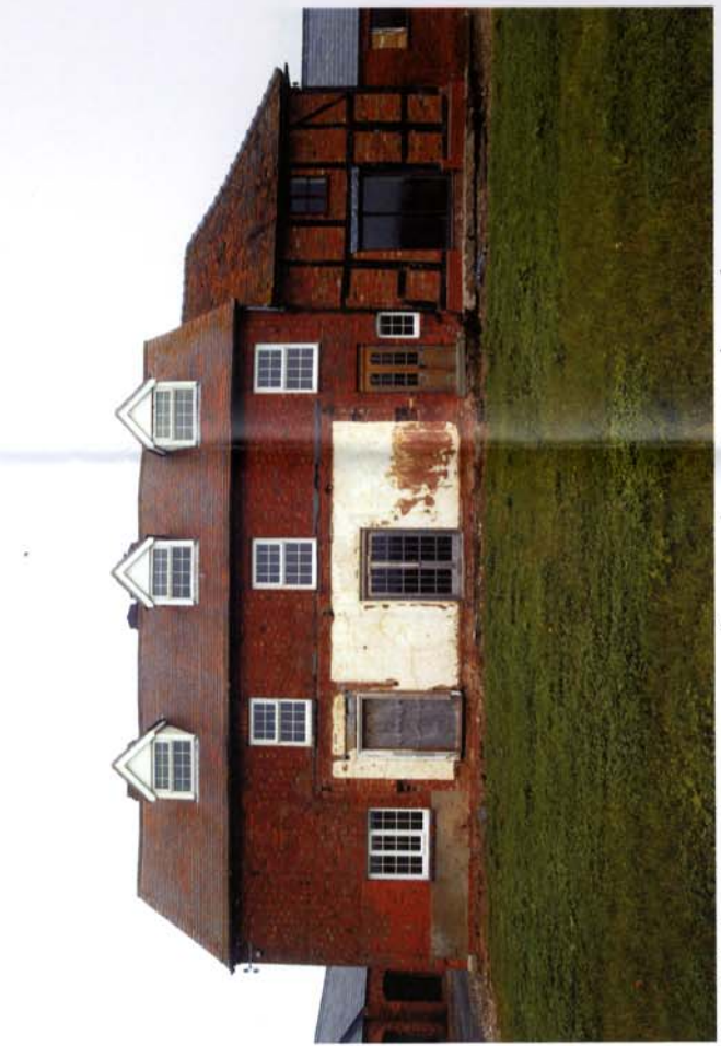
South facing elevation- note scar of removed recent extension and modern plastic windows and dormers
