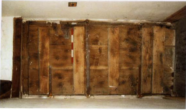
Original door to farm-yard - note surviving door-bar and L 18th C latch
