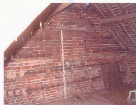
Blocked window in gable end
