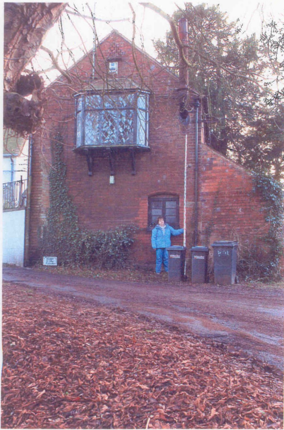
North-eastern gable end - note blocked doorway behind figure
