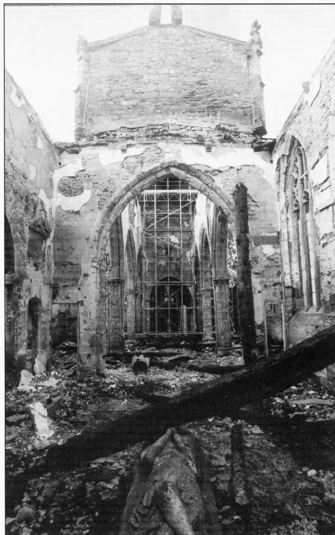
St Brandon's, Brancepeth after the fire, looking west. In the foreground fallen roof beams rest across the 14th-century Peacock of the North effigy. Beyond, the chancel arch and arcades have been seriously damaged by the fire (Photo: Peter F Ryder)
