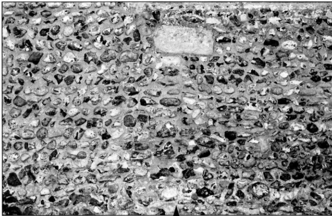
Fig 1 The arrow indicates the straight vertical joint in the nave north wall flintwork, showing the position of the original quoins.
