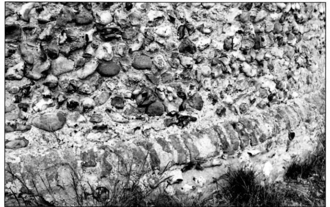
Fig 2 Medieval cant bricks as weathering to the plinth around the base of the tower.
