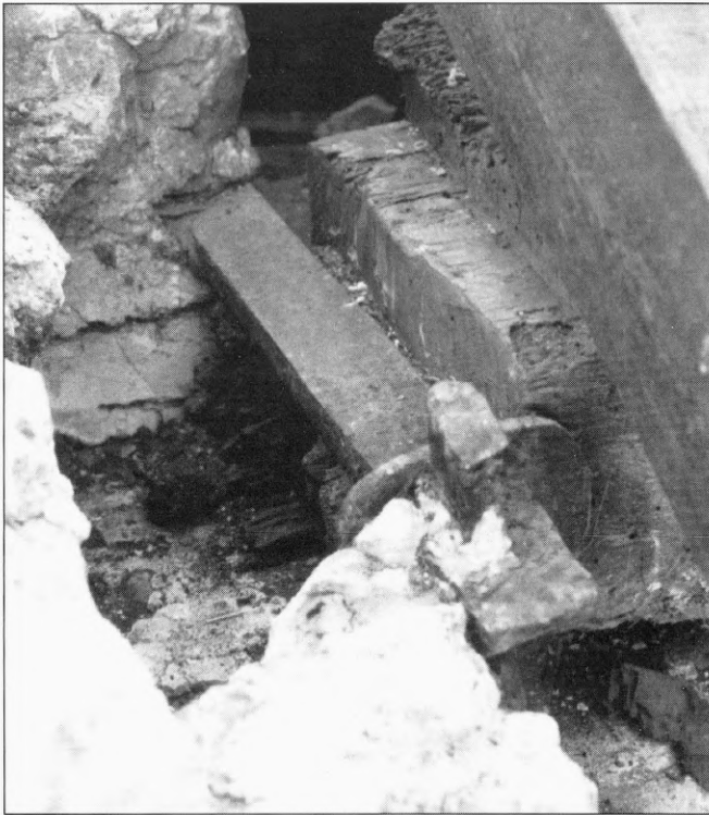
Fig 15: North end of tie-bar in chancel east wall.
