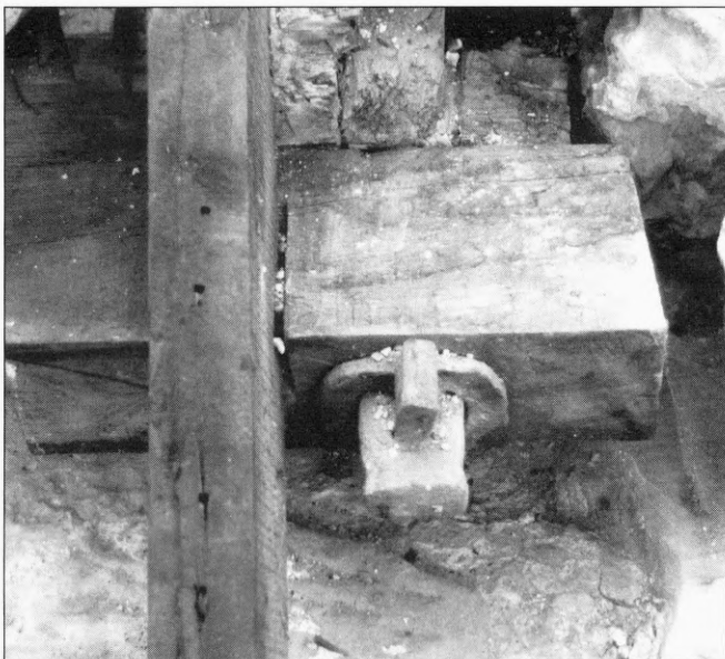
Fig 16: The same tie-bar on south side of chancel.
