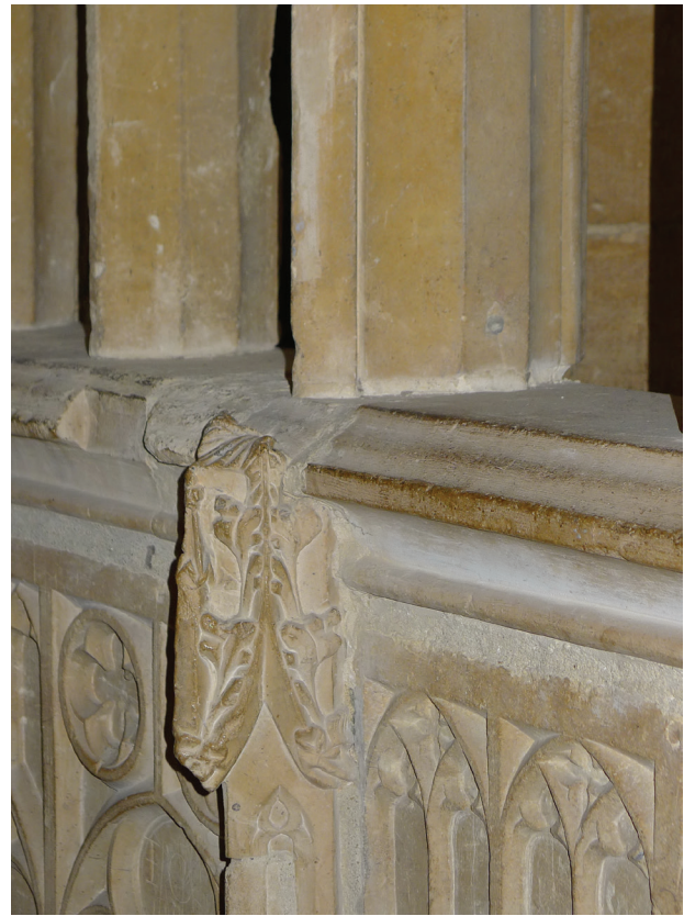
Fig 6 The works chantry screen. Detail of junction between original major mullion and miniature buttress pinnacle rising through dado; dado rail; and later replacement mullion dating from the reconstruction (Photo: author)
