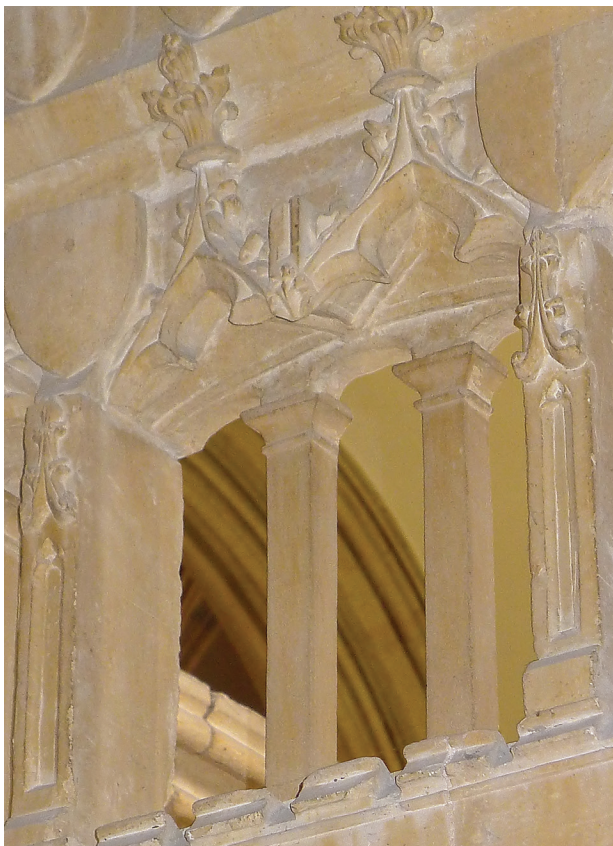
Fig 7 The works chantry screen. Single bay in canopy tier from western side. Note the inserted pillars towards the rear with their 'flared' capitals (Photo: author)
