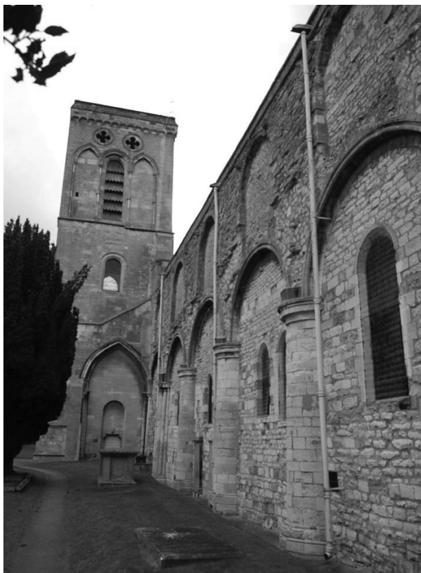
Fig 6 Malton Priory from south, looking west, showing blocked arches of nave arcade and gallery and roof weathering on tower (Photo: author)
