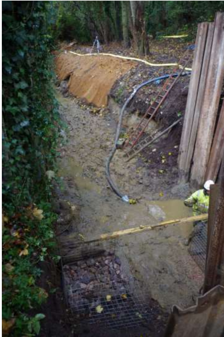
Plate 1. Work in progress in November 2015 at the commencement of the watching brief. The southern part of the excavation has been completed and the sides lined with textile to prevent erosion. The natural Wittering Formation can be seen in the base and side of the excavation. The trench was not safe to enter.
