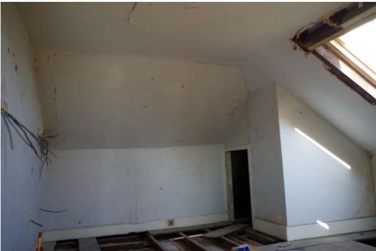
Figure 11. View of north part of attic showing typical construction before opening up.
