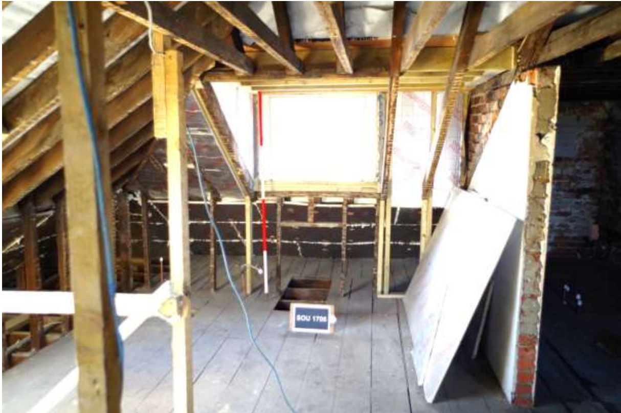
Figure 16. View showing studwork in the attic after removal of lath and plaster.
