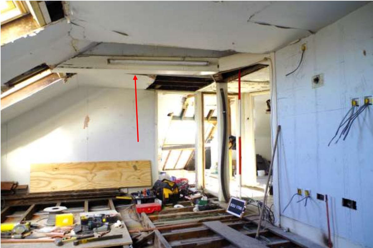
Figure 10. The attic space on first visit. Red arrow points to the boxed-in lead pipe.
