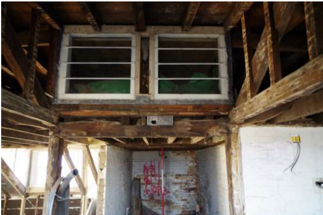
Figure 13. The window openings (with more recent frames and bars) in the east wall of the flat roof/light well, with lead hopper beneath them, after removal of the lead pipe, supporting beam and its enclosure.
