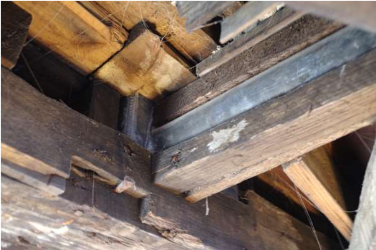
Figure 14. The base of the lead hopper, with lead pipe exiting to the right (east). Note housing with protruding nail below the hopper which probably relates to an earlier layout of the attic space.
