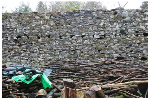
Fig 17. Building 1 b joist holes.
