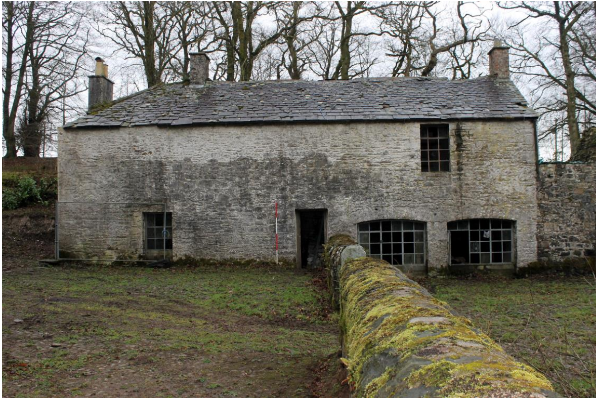
Fig 34. Building 5 from NW showing 5a (right), courtyard wall, entrance to 5b (centre), entrance 5c (left) and window to cottage living room 5d (above right).
