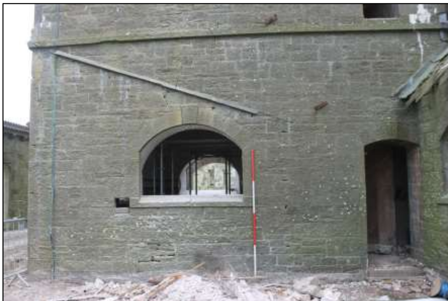
Plate 18. Tower, ground floor west face showing entrance to stairs and roofline of former building.
