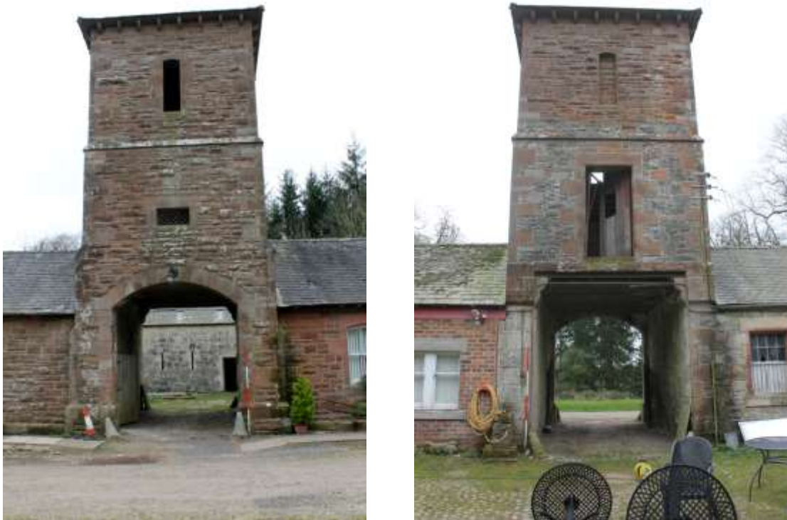
Fig. 20. East Wing – EW3 pend and tower (left: outer face; right: inner face).
