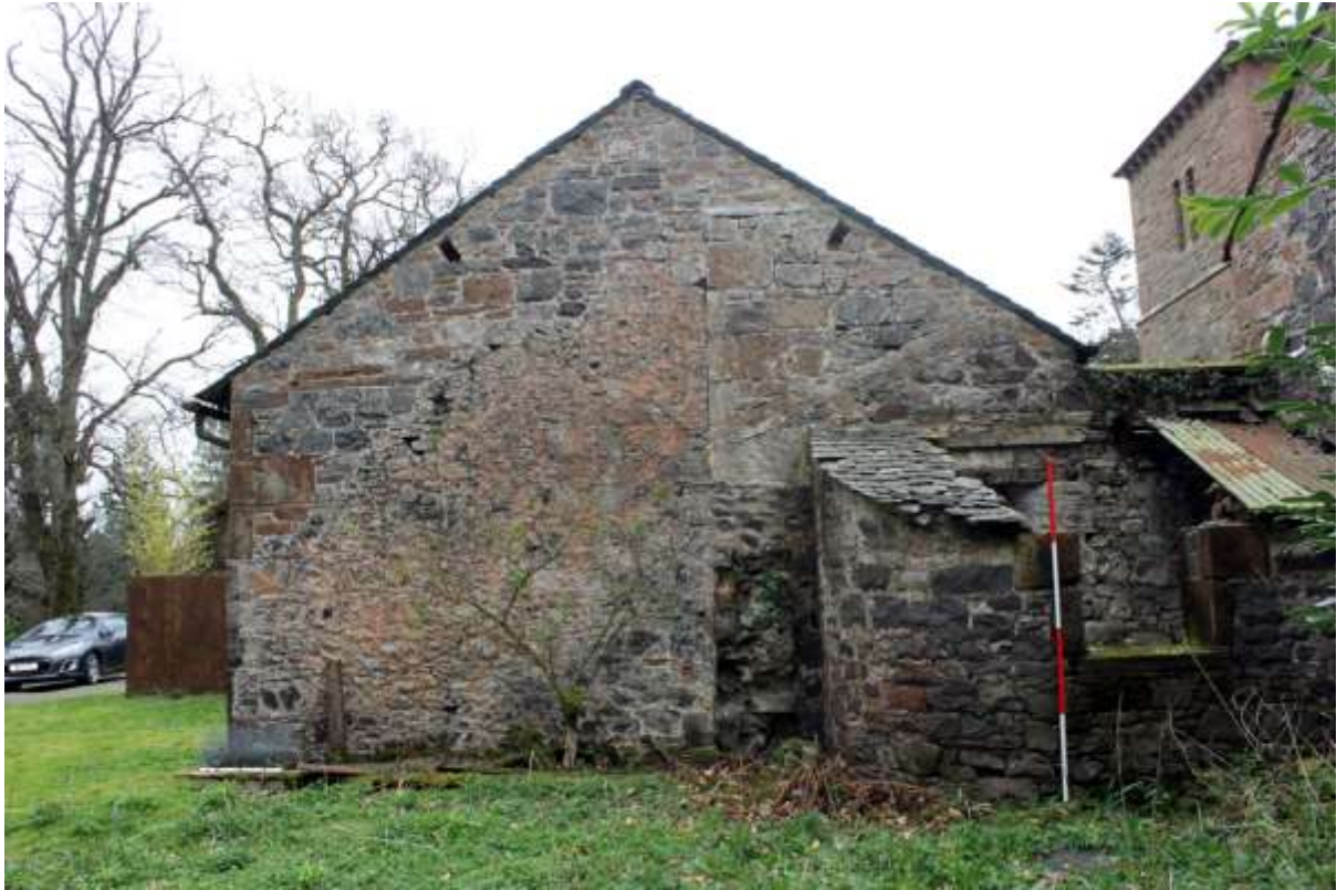
Fig. 10. West gable wall showing building phases. The angled slots are for the Phase 3 roof purlins.
