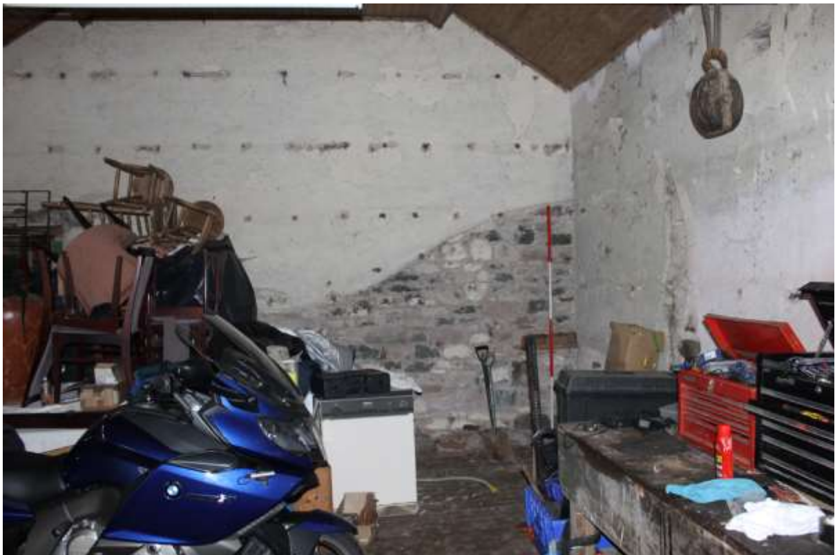
Fig. 11. Interior view showing outline of stable stall and support holes for wall panelling.
