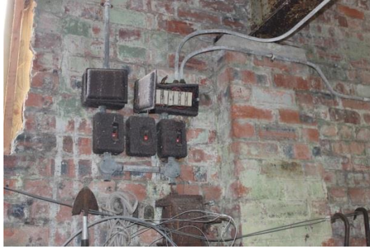
Fig. 13. Building 1, electrical junctions + conduits.
