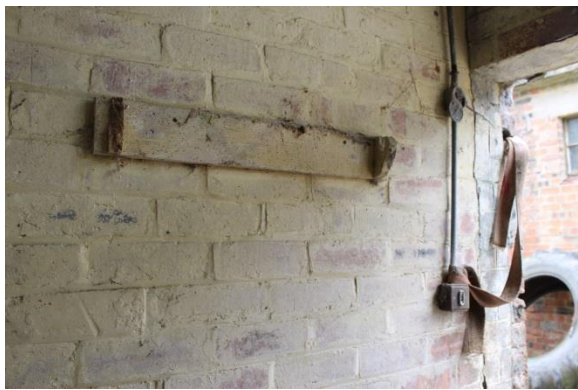
Fig.21. Building 2, towel rail in toilet block 2c.
