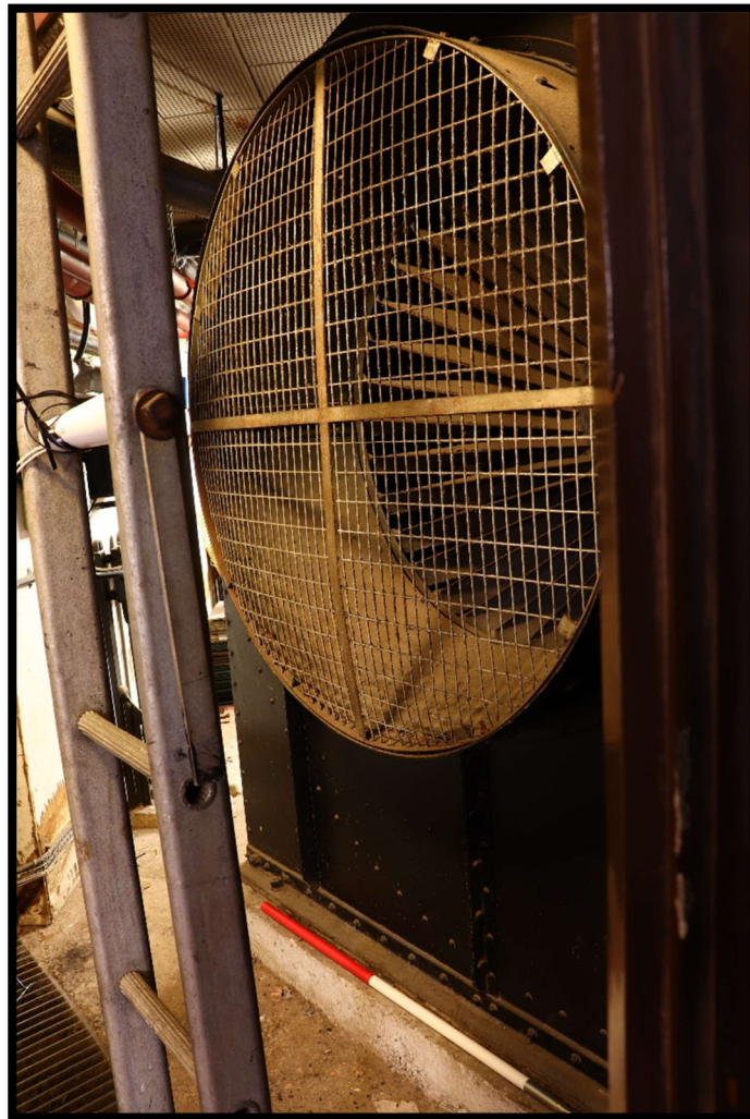
Figure 1 basement - 1930s heating ventilation fan, scale 1m
