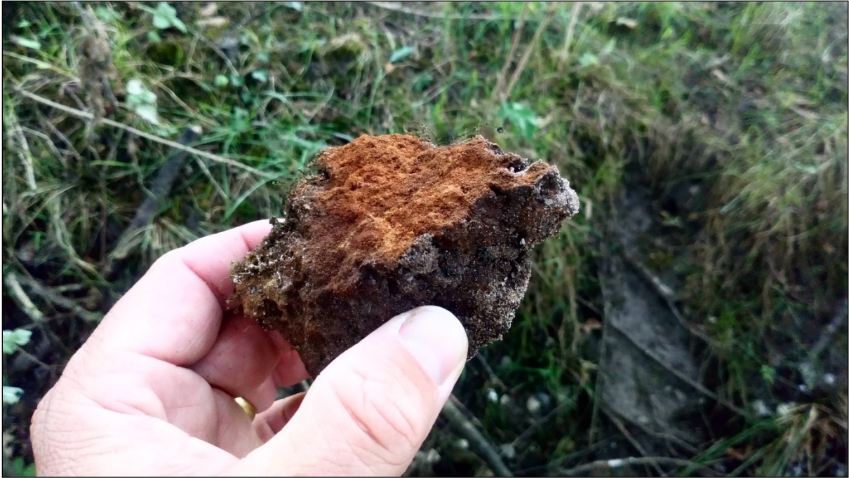
Figure 26 Sandy stone material eroding from the edge of the pond
