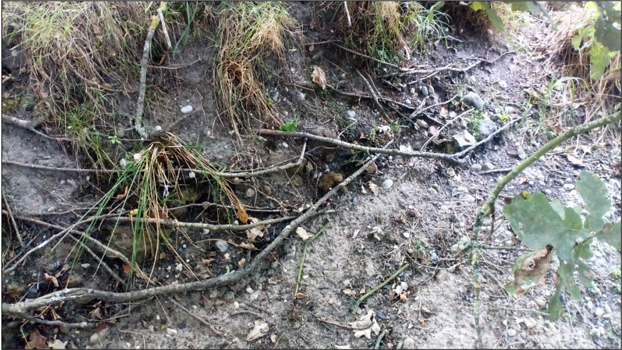
Figure 24 Material eroding from the side of the pond along its western edge
