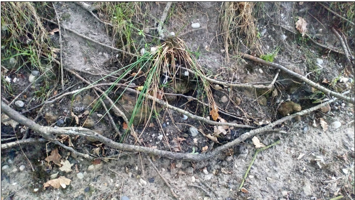
Figure 25 Detail of in situ sandy material eroding from the side of the pond
