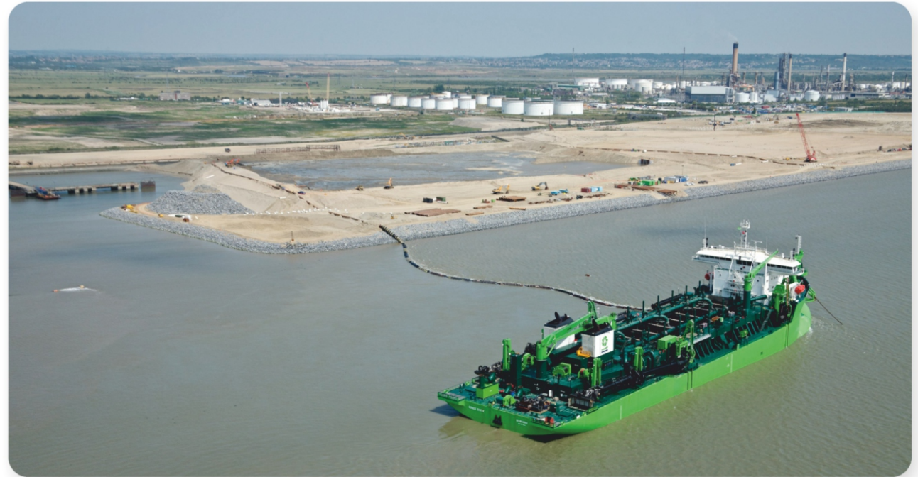
The Congo River unloading dredged material into the reclamation areas during the construction of DP World London Gateway Port
