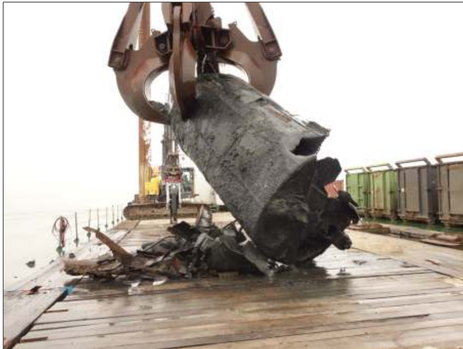
Plate 1: Boiler, WA3007, held within the grab's teeth having been recovered from the site
