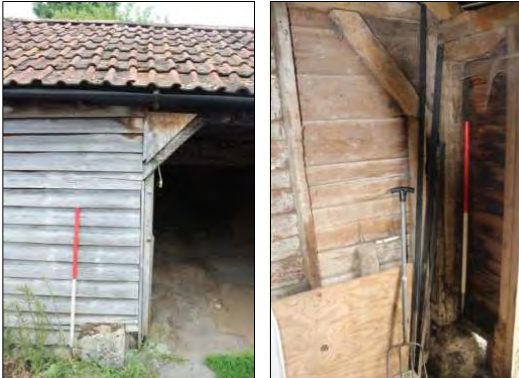
Photos 29 & 30 External view of Frame C, noting the brace (left) and internal view of Frame B (right)
