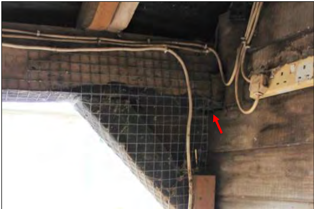
Photo 39 Detail of the post on the south end of Frame C, with junction identified by red arrow
