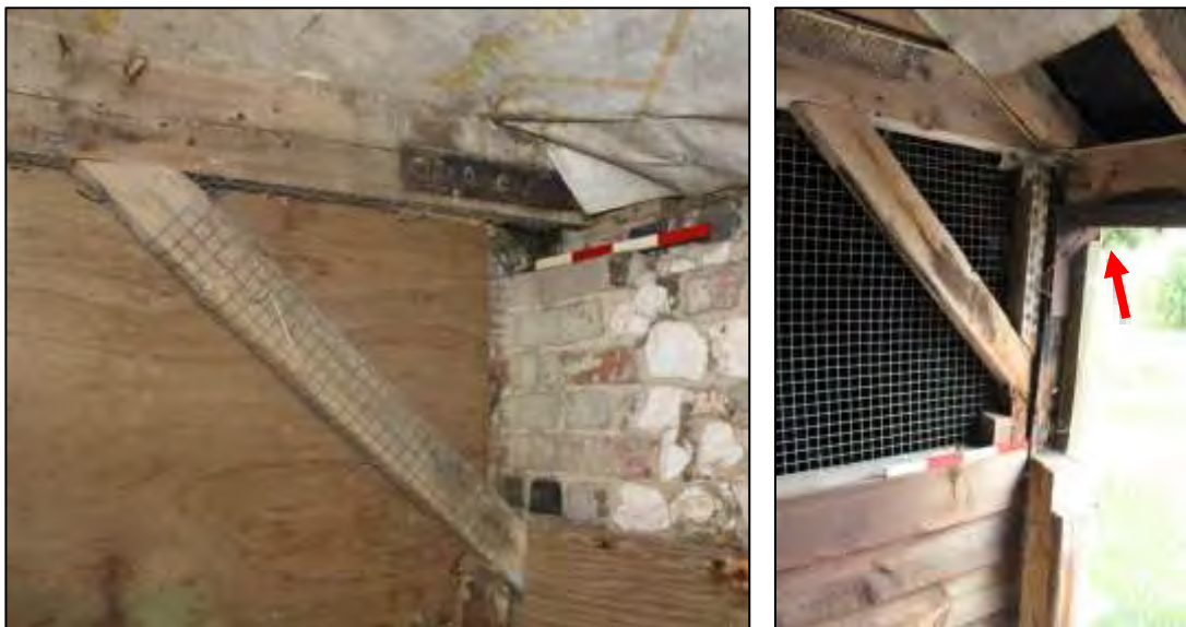
Photos 40 & 41 North end of Frame D (left) and south end of Frame E from Bay 4 (right)
