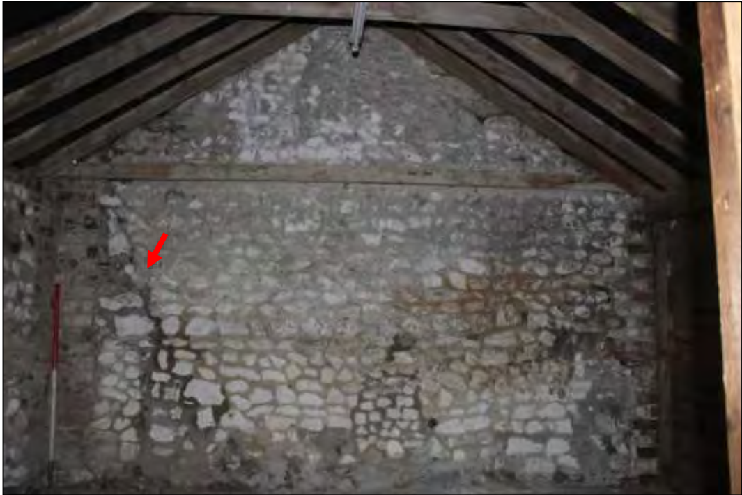
Photo 44 Internal view of East masonry wall, with crack location identified by red arrow
