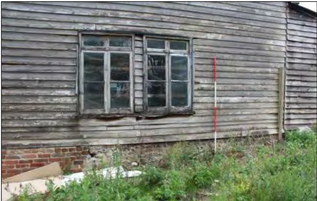
Photo 52 Detail at west end of the Warehouse, note the various materials of the plinth
