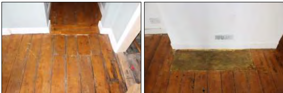
Photos 19 & 20 Stained floorboards contrasting with the unstained boards in the airing cupboard (left) with stain carried over the hearth (right)
