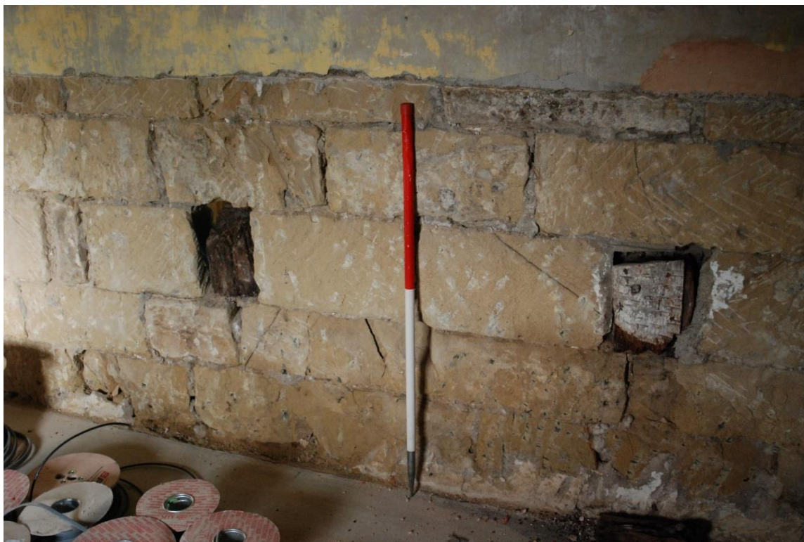
Plate 3: Detail of timber blocks (MH04 and MH05) within the wall between kitchen and living room. Facing north-east.
