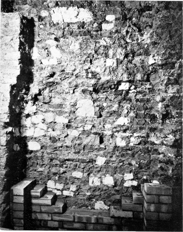
Fig. 5.—NORTH WALL OF THE SERVANTS' HALL OF THE PRIVATE HOUSE OF THE TIMES OFFICES.
