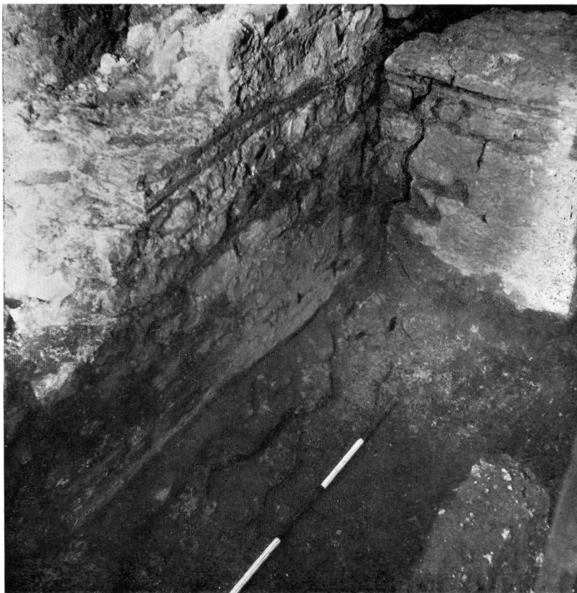
PLATE C. Junction of Roman city wall ( left ) and north wall of internal turret ( right ), showing the crack where the former has pulled away from the latter. (Scale in feet).
