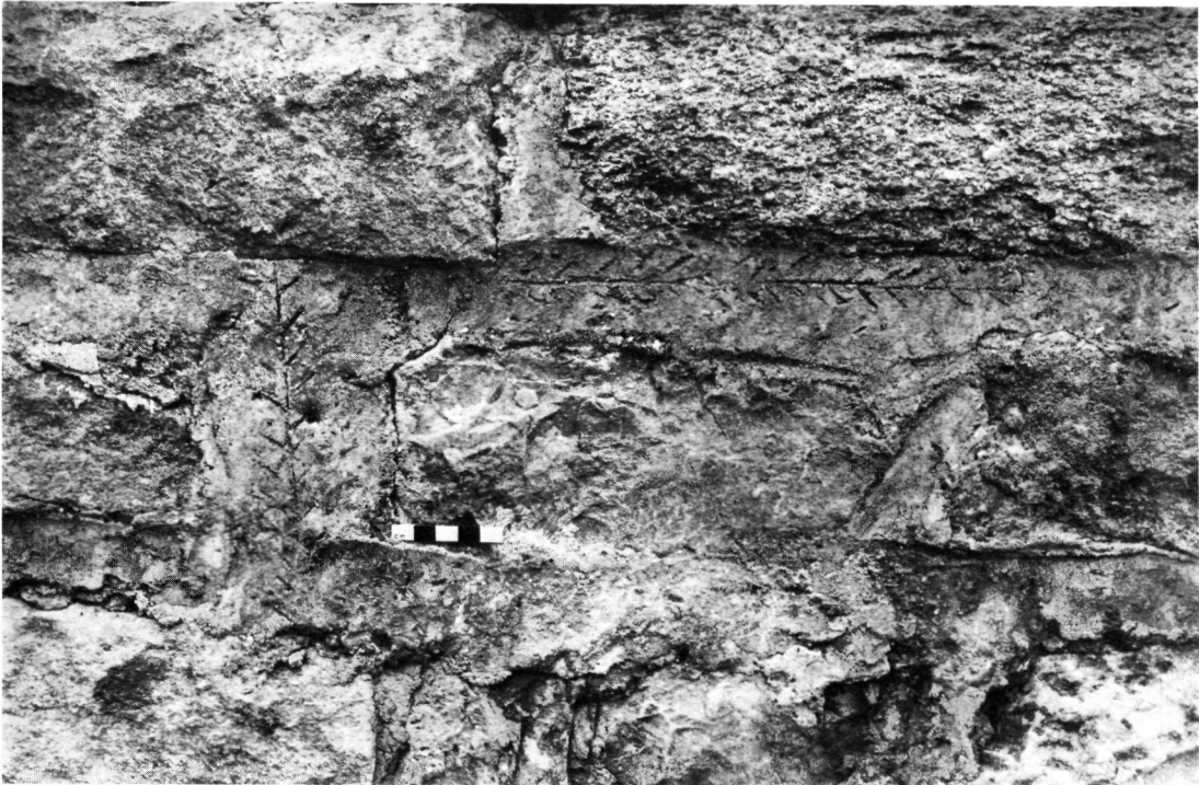
Plate 10 Inmost Ward 1977: Detail of pointing on north (landward) face of late 4th-century riverside wall showing incised herringbone design (5cm scale).
