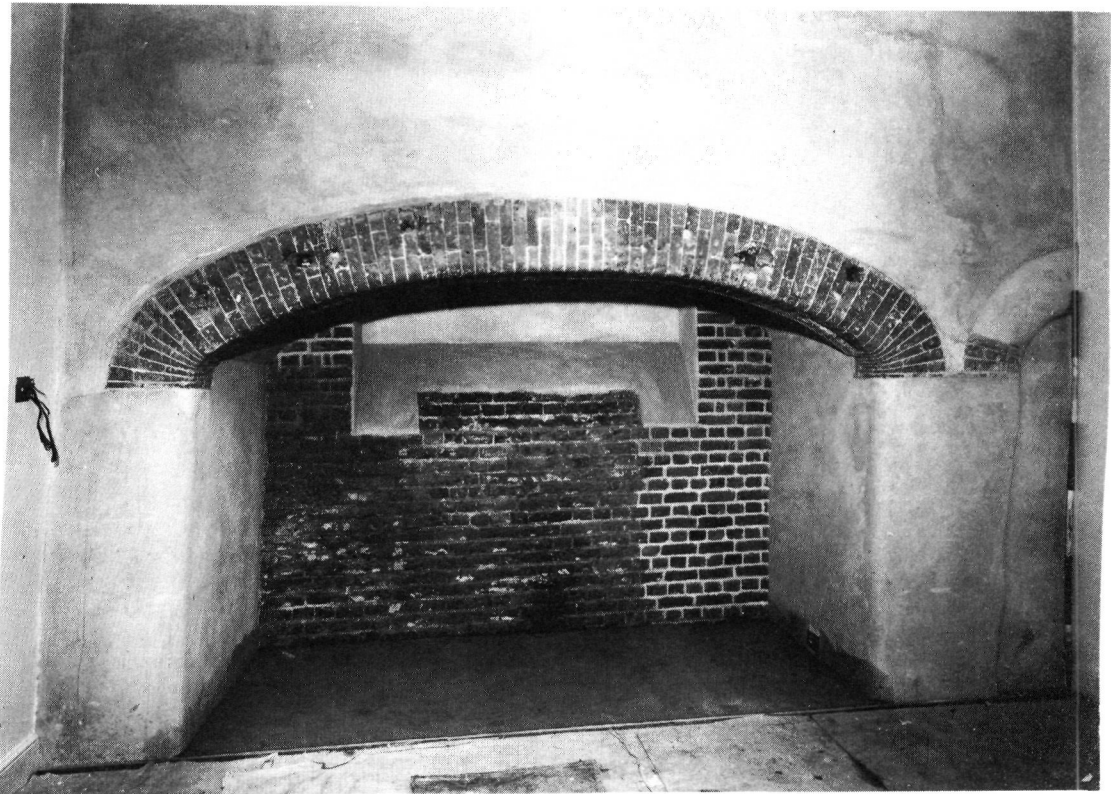
Plate 39 Reconstructed fireplaces in the kitchen of the Duke of Monmouth's lodgings (Crown Copyright)
