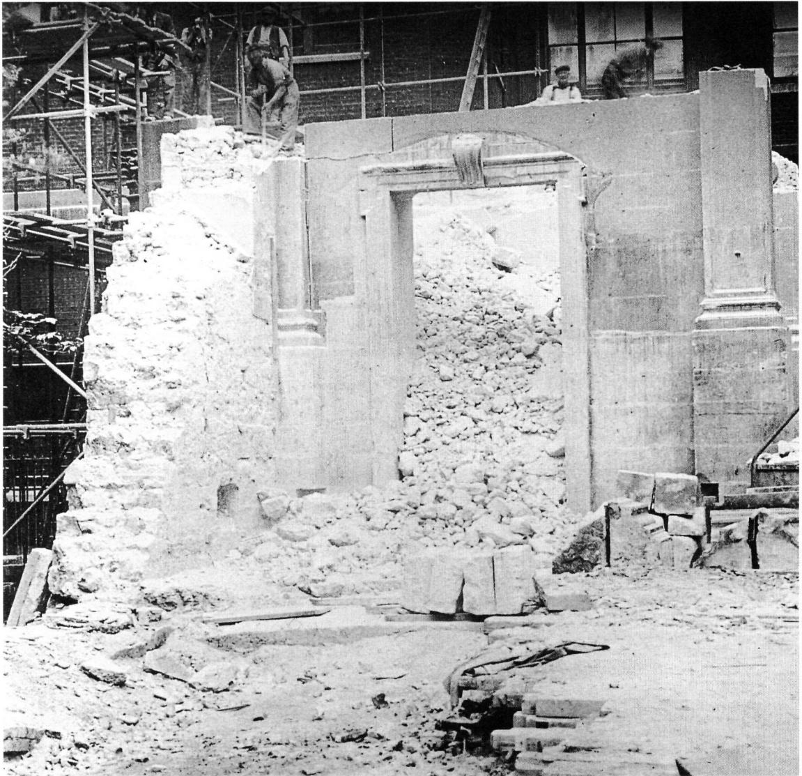
Fig 53. All Hallows Lombard Street (6): demolition of the west end of the Wren church in progress, 1939 (GM)
