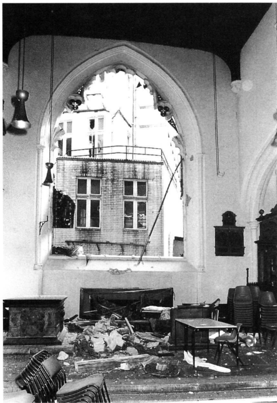
Fig 67. St Helen Bishopsgate (44) : the north aisle window blown in by the bomb of April 1992. It has now been replaced by a new window
