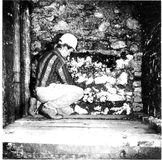
Fig 11. West face of west wall of St Ethelburga’s Church, seen at the end of the header trench
