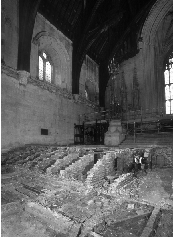
Fig 18. Westminster Hall: view looking south-east, showing Smirke's sleeper walls and floor slabs and the arched support walls for the 1850s south steps
