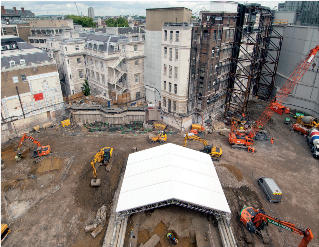
Fig 3. Site B excavation trench, covered by a moveable roof for weather protection, looking north
