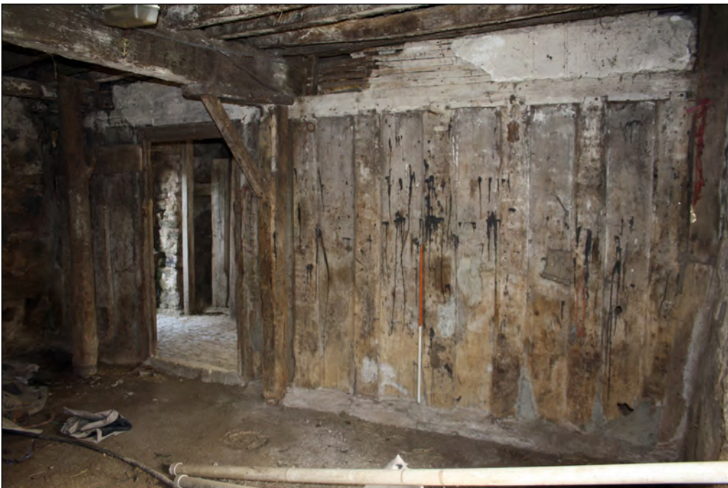
Plate 8. South screen, facing north, 1m scale
