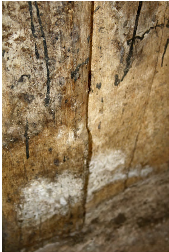
Plate 10. Worn chamfer on south screen, south elevation
