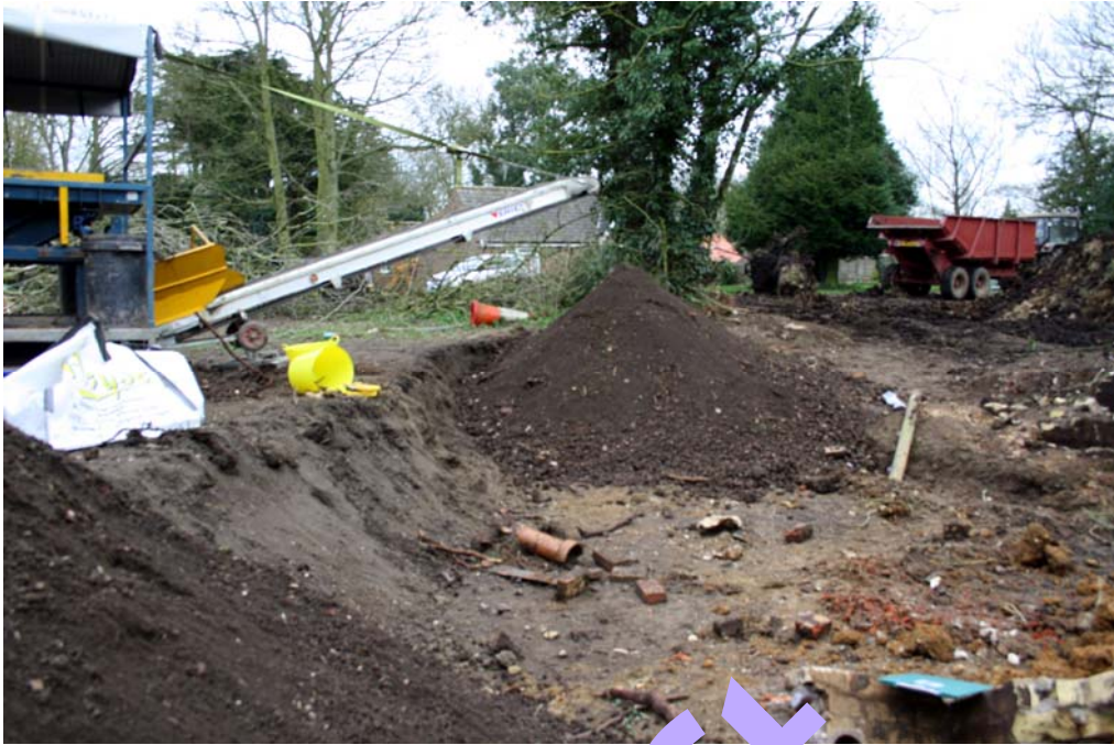
Plate 4. Spoil heap created by the return of screened soil to site (from which the finds were recovered)
