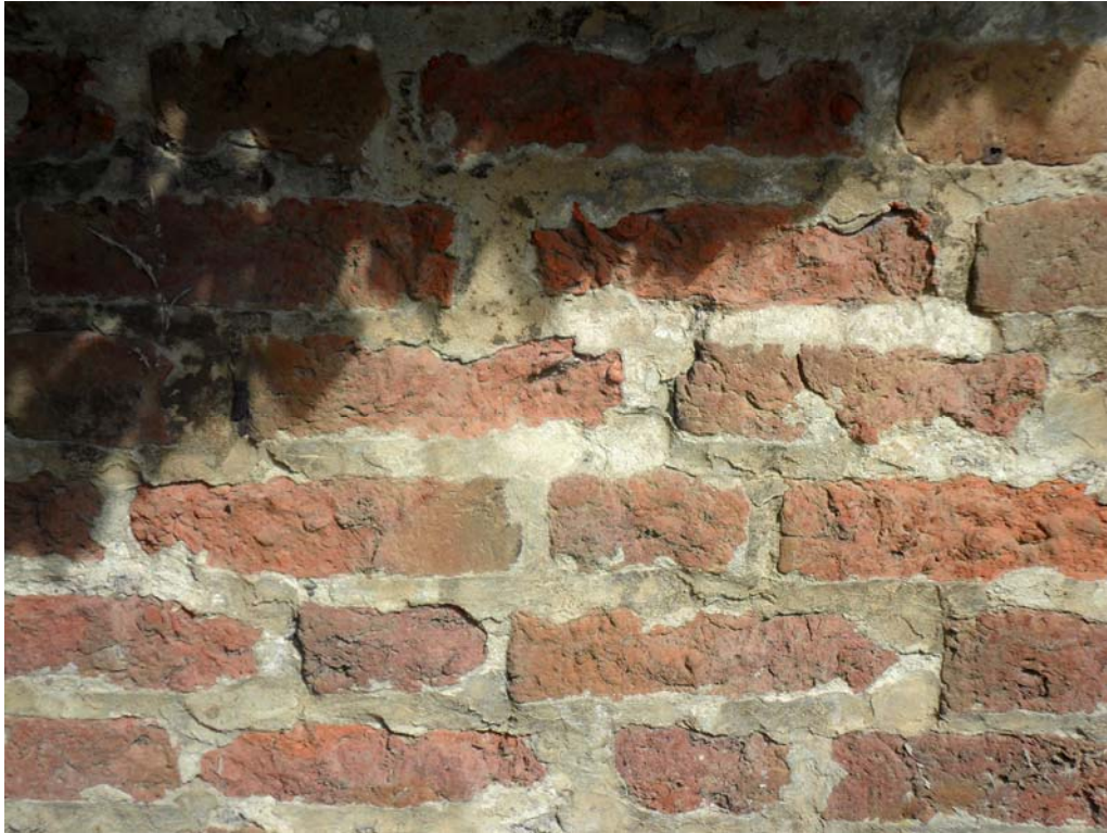
Plate 16. The main brick types in the exterior wall; a pinkish red brick and a browner brick (visible at top right)
