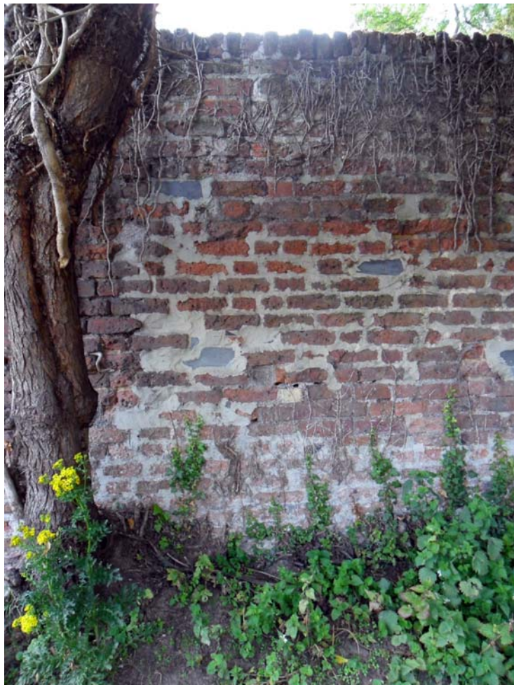
Plate 15. Typical example of the interior of the wall, showing heavy patching, looking west
