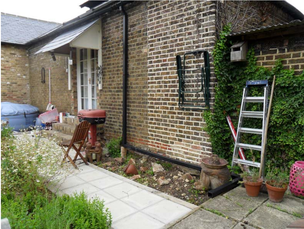
Plate 13. Building 2, exterior west side showing new doorway and modern extension to the left
