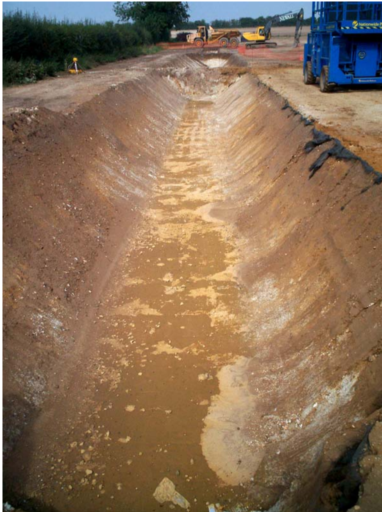
Plate 4: Infiltration Trench B, facing east
