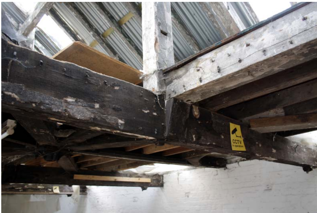
Plate 13 Detail of connection of queen post to the tie beam and cart wheel roof structure
