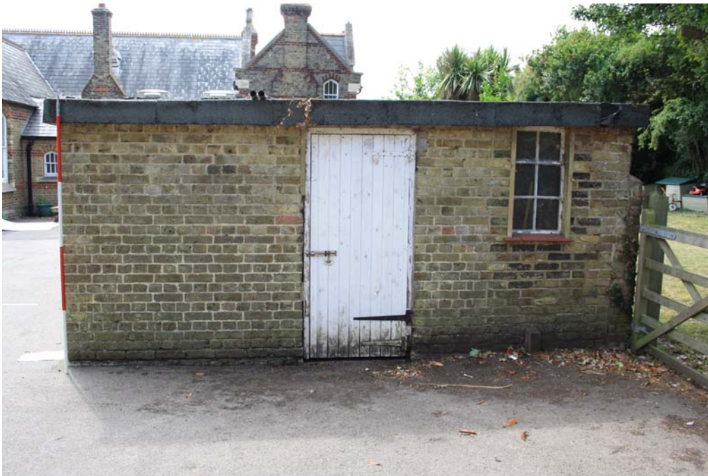
Plate 3. The north-west wall showing the later door and blocked original door occupied by the later window
