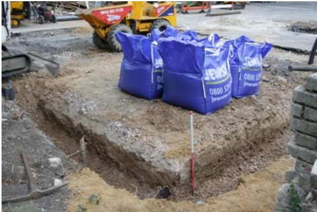
Plate 7. View north across the excavations for the foundations of the new hall
