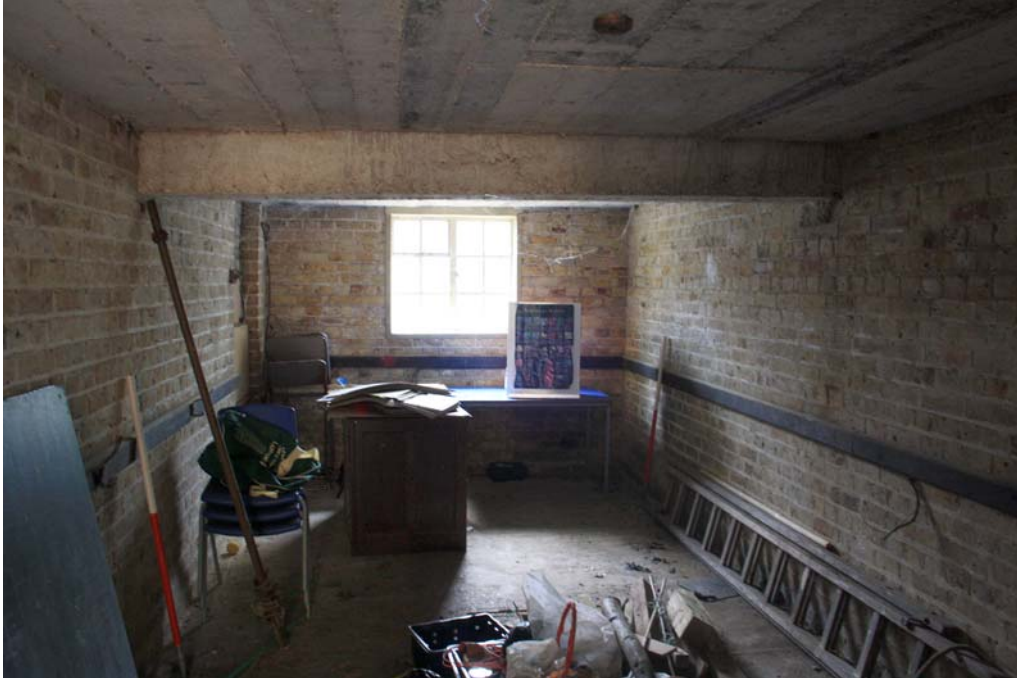
Plate 5. Interior of Room 2 showing later window and the impressions of the timber shuttering in the poured concrete roof
