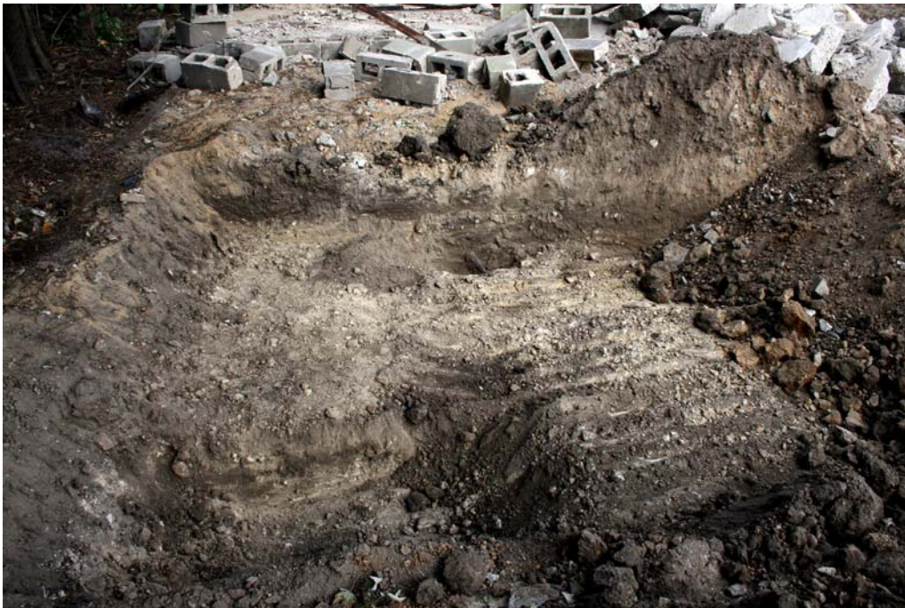
Plate 1. General view north across the watching brief area showing the chalk natural and the modern features cutting through it
