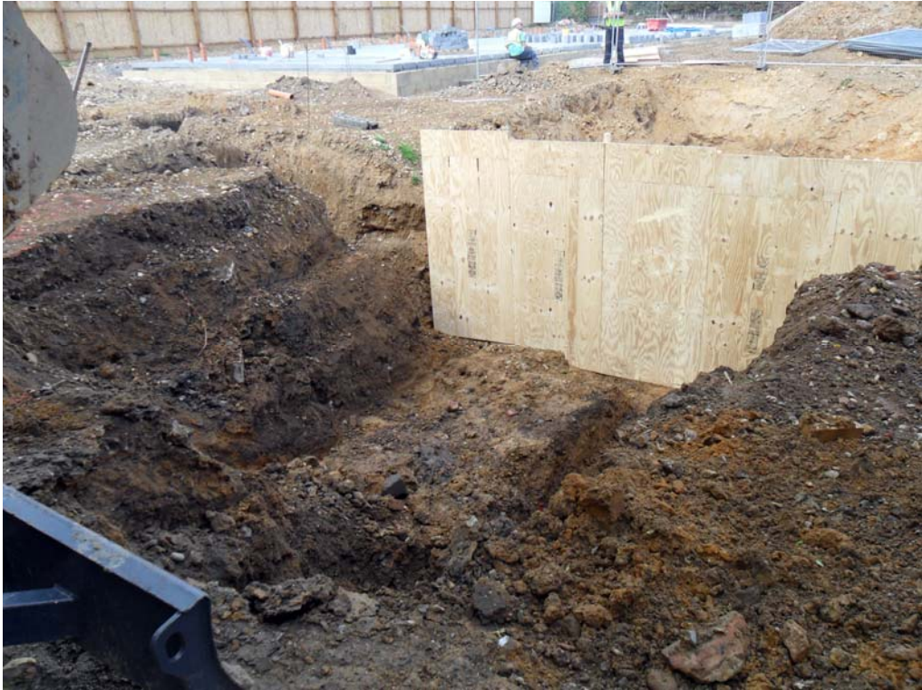
Plate 3. Slippage caused by excavations close to the old cellar
