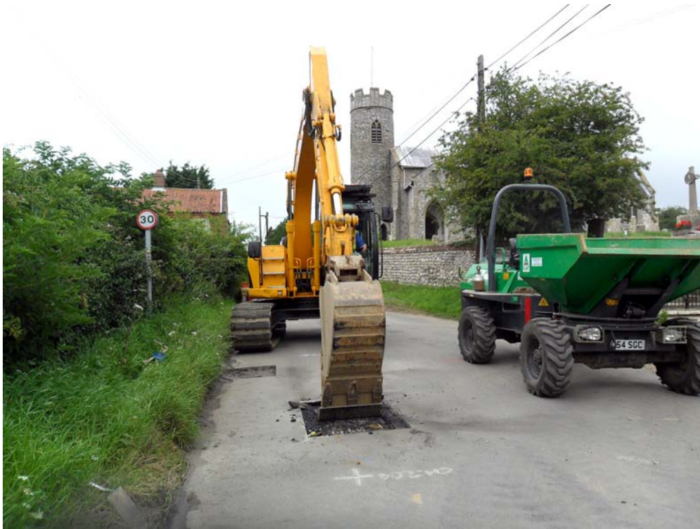
Plate 1. Excavation of trench in roadway (St John the Baptist's church in the background)
