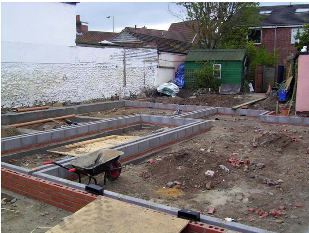
Plate 1. General view south-west across the site following the construction of the new foundations
