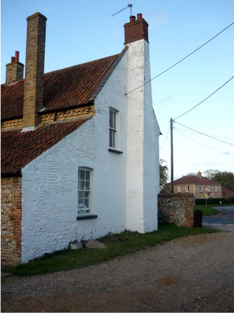
Plate 4. The south-east gable wall showing the location of the proposed new soil pipe
