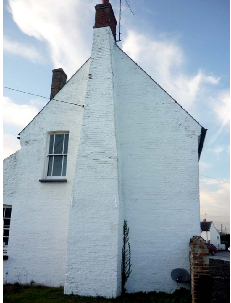
Plate 5. The south-east gable wall showing the location of the proposed new vent
