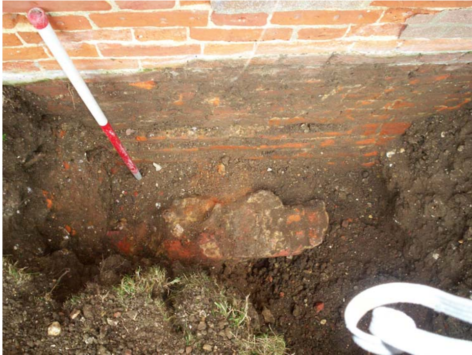
Plate 5. Base of south-west facing elevation of 'kitchen' showing stepped foundation of wall [4] and the remains of demolished 'wall' [2]; looking down test hole.
