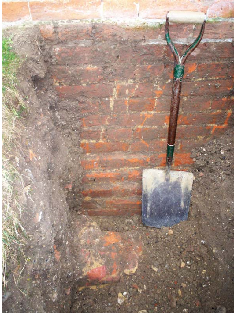
Plate 4. Base of south-west facing elevation of 'kitchen' showing stepped foundation of wall [4] and the remains of demolished 'wall' [2]; facing north-east.
