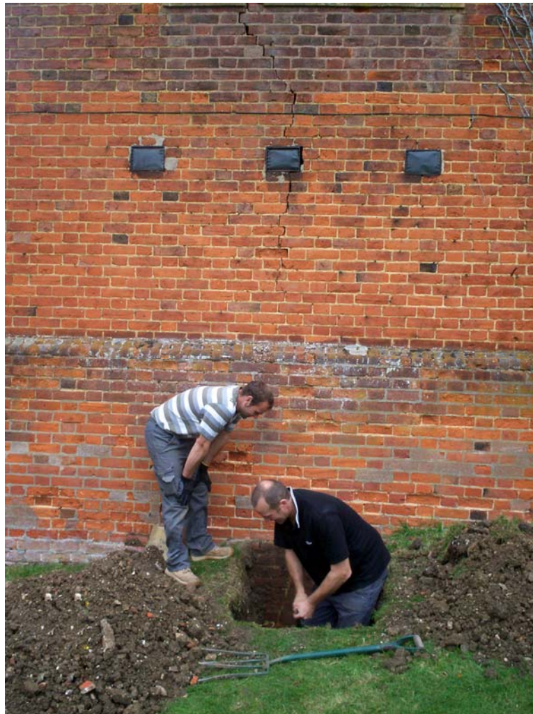
Plate 2. South-west facing elevation of 'kitchen' with test pit being excavated by staff of Brown and Ralph. Photograph indicating depth of hole; facing north-east.
