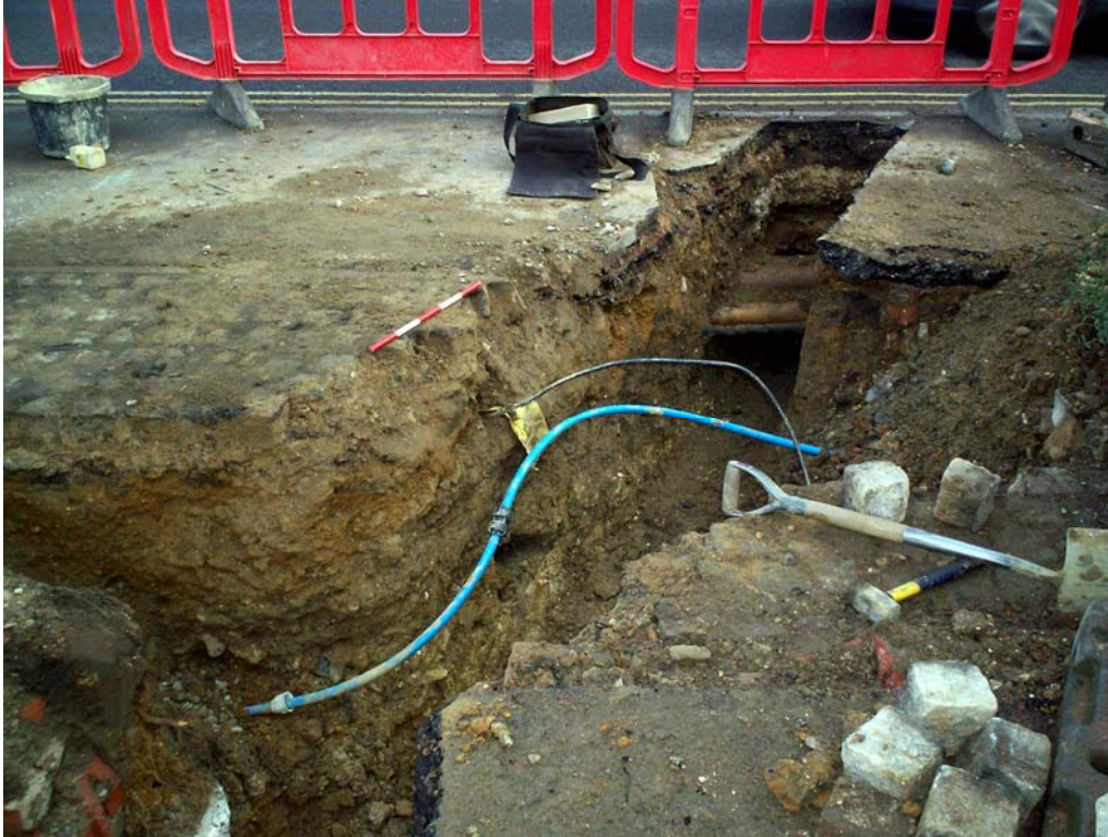
Plate 2. Pipe trench looking east (with the existing manhole at the eastern end of the trench beneath the wheel of the passing car)
